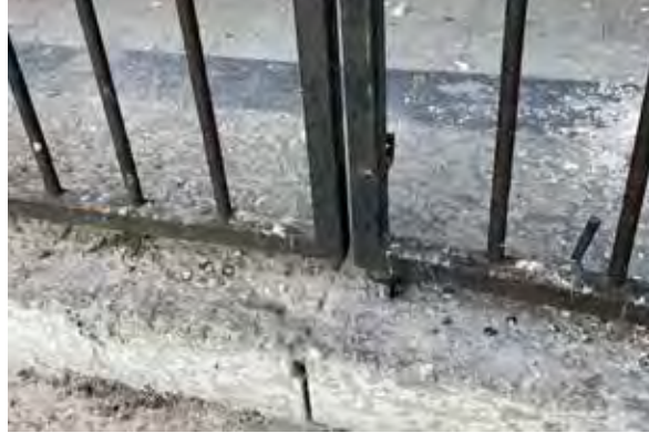
Fig. 26. Damage and staining to steps.
