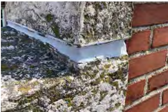
Fig. 59. Pitting, staining and organic growth on parapet.
