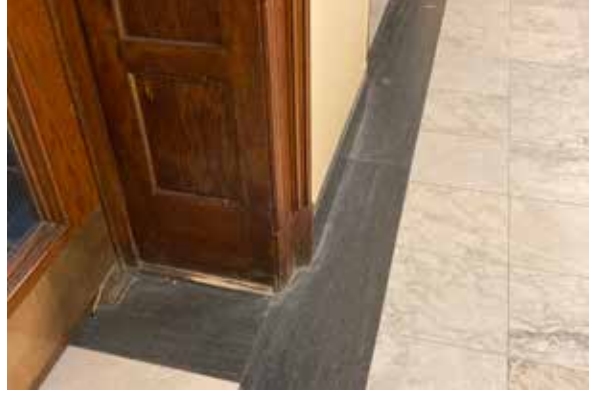
Fig. 97. Main lobby surface wear.
