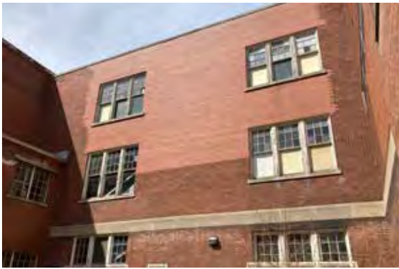
Fig. 53. Unsympathetic window replacements.
