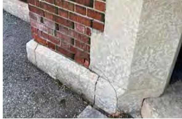
Fig. 5. Example of efflorescence towards base of exterior.
