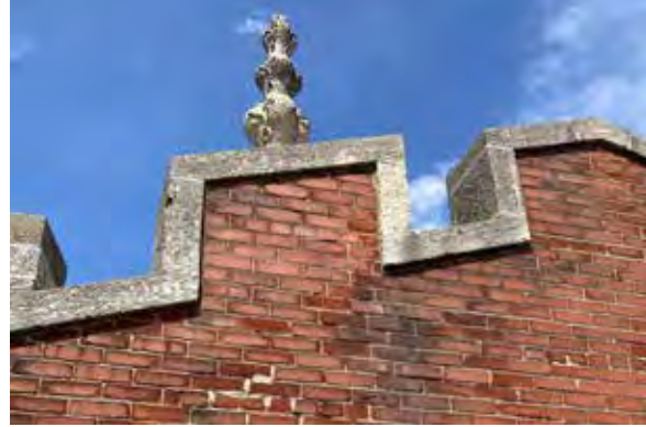
Fig. 66. Area of stone degradation and chipping.
