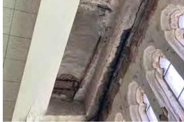
Fig. 110. Deteriorated cement finish.
