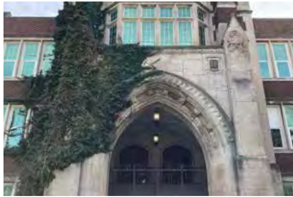
Fig. 28. Growth on the tower impeded proper inspection.
