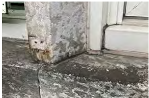
Fig. 15. Example of stone staining, holes and rust.
