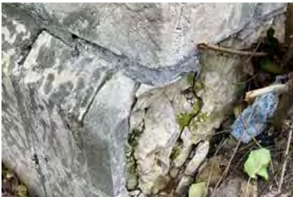
Fig. 25. Large cracks at base of pilasters.
