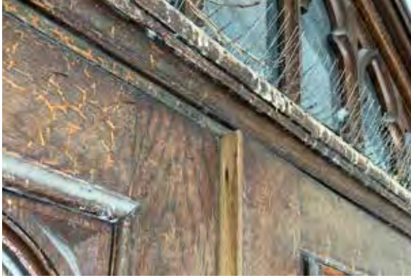
Fig. 81. Cracking of wood coating.
