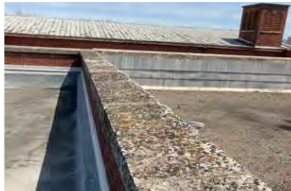
Fig. 63. Pitting, staining and organic growth on parapet.
