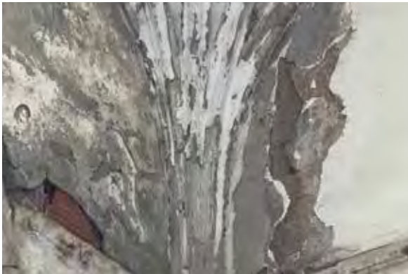
Fig. 35. Local deterioration to to stucco and rib elements.
