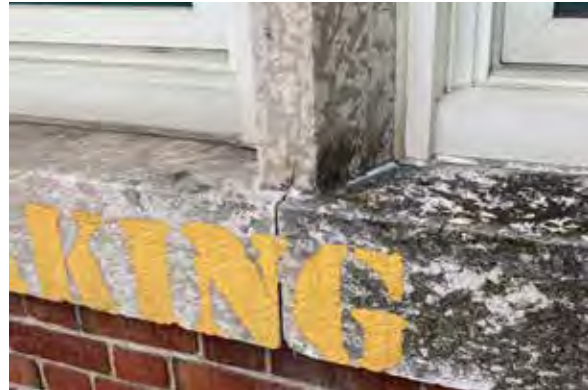
Fig. 20. Example of overpainting on exterior sills.
