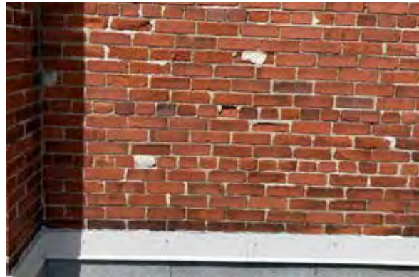
Fig. 67. Evidence of spalled brick and Incompatible repairs.
