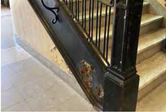
Fig. 106. Corrosion at base of west stair.
