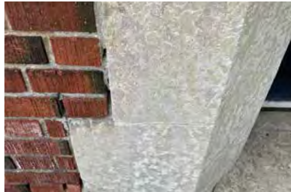
Fig. 8. Recessed mortar joints between stone and brick.
