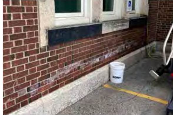
Fig. 18. Example of overpainting on exterior sills.
