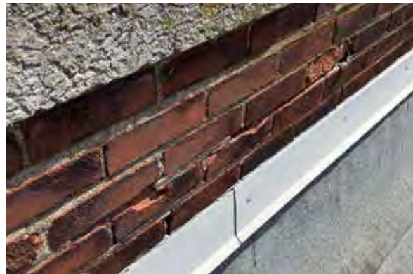
Fig. 68. Chips and spalled brick.
