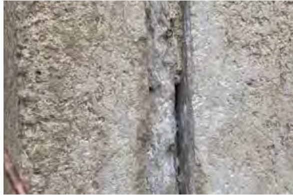
Fig. 27. Evidence of patch repair damage to stone.
