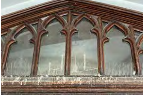
Fig. 82. Bird droppings on otherwise intact transom.
