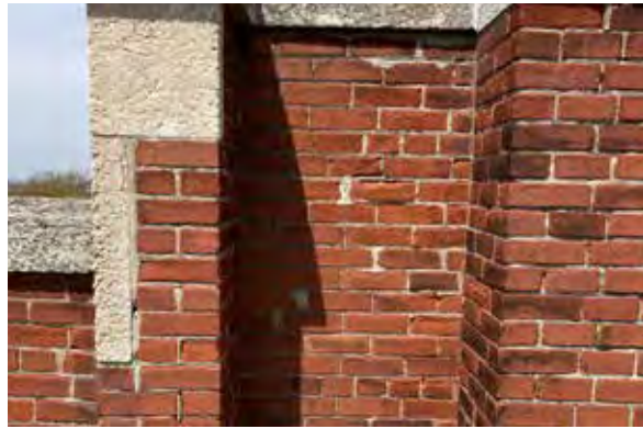
Fig. 75. Incompatible brick replacement (left).
