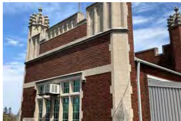
Fig. 32. Growth on the tower impeded proper inspection.
