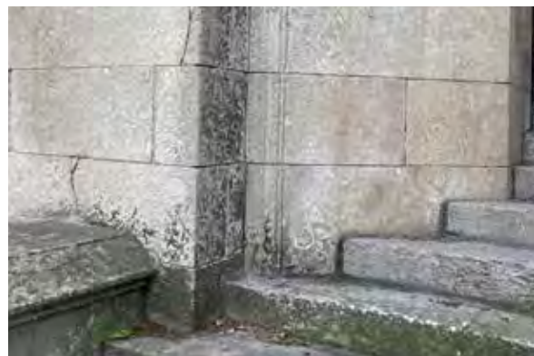
Fig. 21. Eroded stone joints & organic growth.
