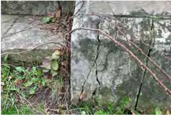
Fig. 23. Large cracks at base of pilasters.
