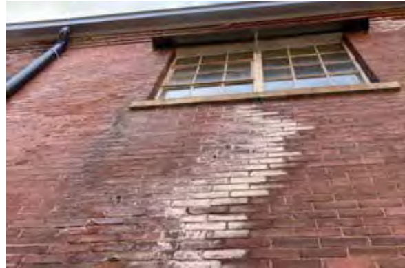
Fig. 47. Severe efflorescence and some spalling.
