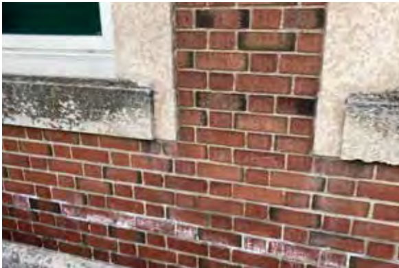
Fig. 4. Example of efflorescence towards base of exterior.
