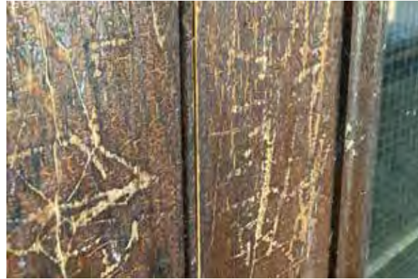
Fig. 77. Surface scratching of northern entrance door.
