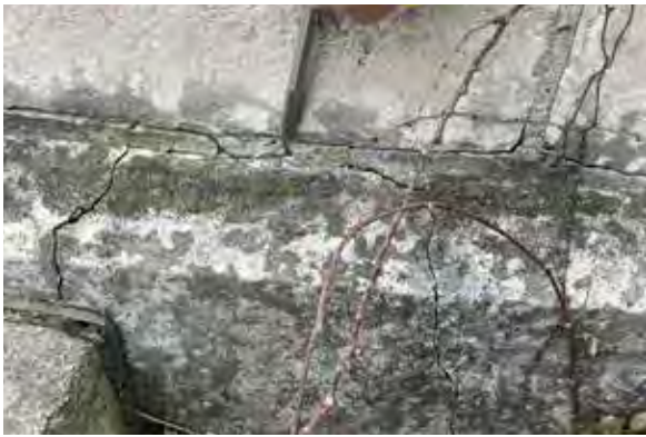
Fig. 24. Large cracks at base of pilasters.
