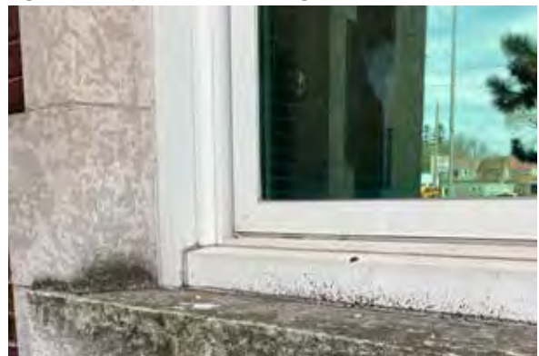
Fig. 16. Significant stone staining and organic growth.
