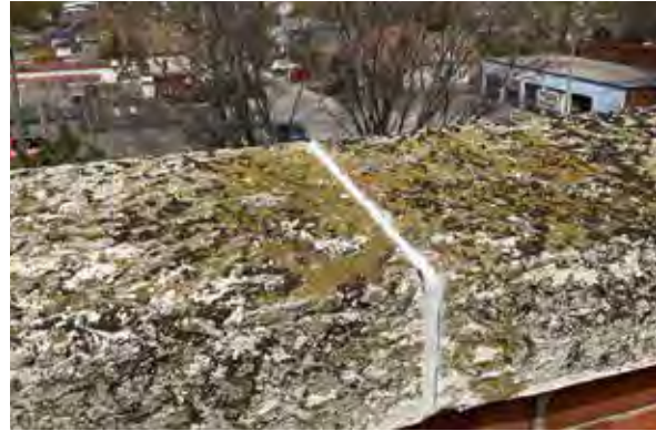
Fig. 60. Pitting, staining and organic growth on parapet.
