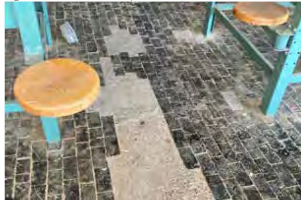
Fig. 116. Block flooring concrete patches.
