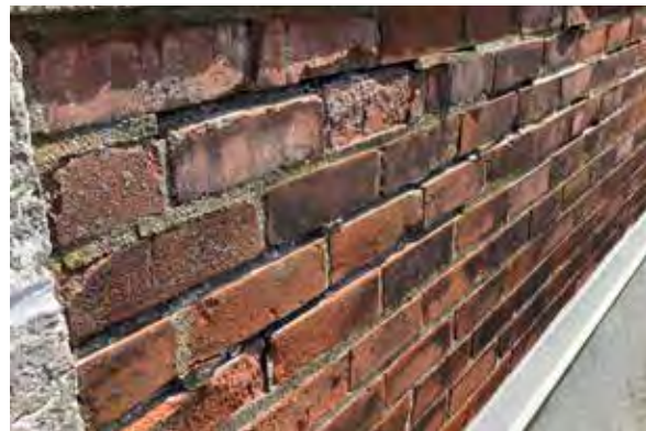
Fig. 69. Spalled brick and loss of mortar joints.
