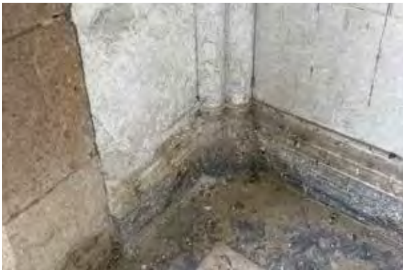
Fig. 36. Soiling at base and floor.
