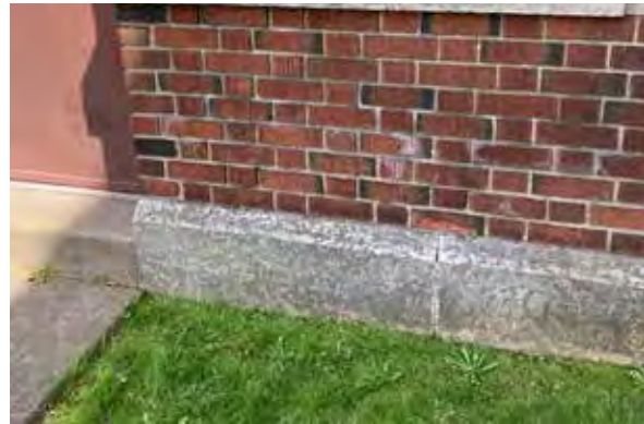
Fig. 6. Example of efflorescence towards base of exterior.
