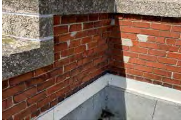
Fig. 74. Incompatible spall repair.
