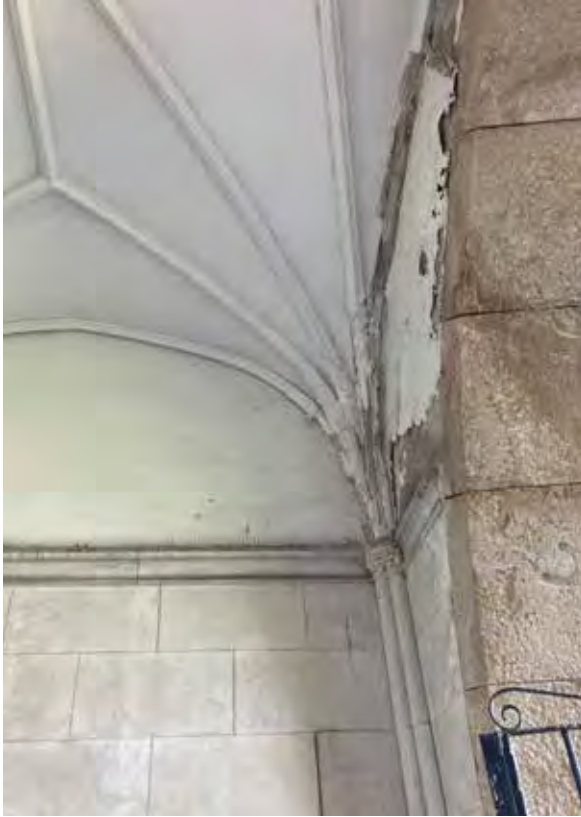
Fig. 34. Local deterioration to to stucco and rib elements.
