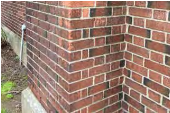
Fig. 2. Example of minimal spalling.
