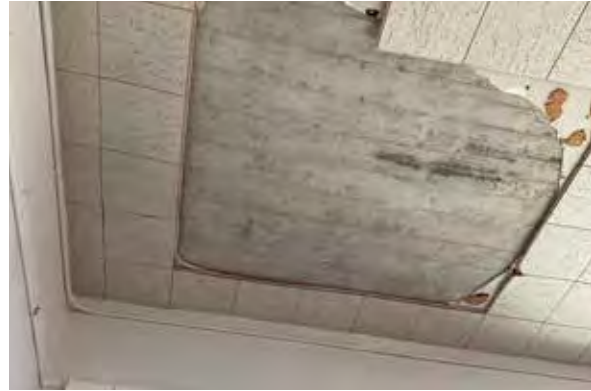
Fig. 111. Missing ceiling tiles and exposed roof deck.
