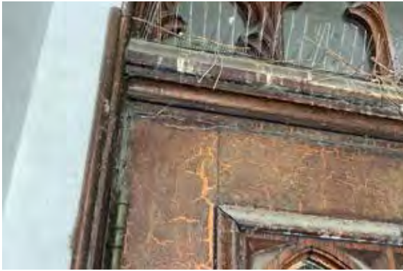
Fig. 83. Broken section of moulding below transom.
