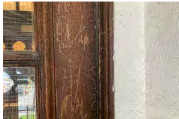
Fig. 79. Surface scratching of northern entrance door.
