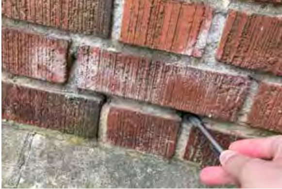
Fig. 9. Recessed mortar joints.
