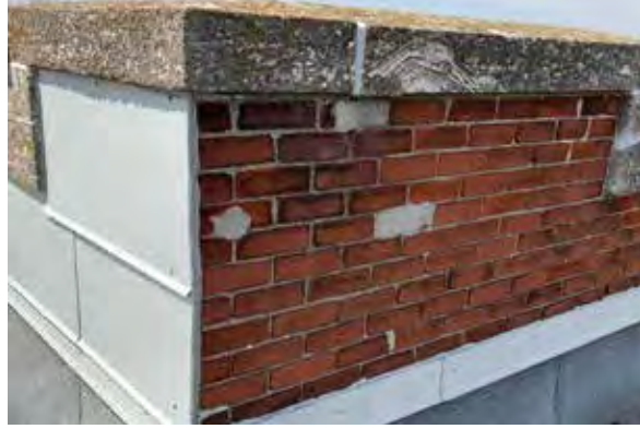
Fig. 73. Incompatible spall repair.
