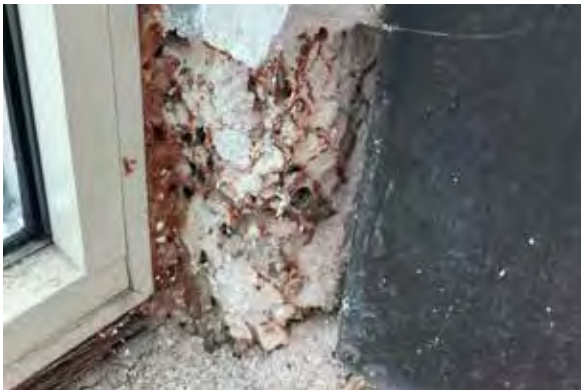
Fig. 108. Failed concrete sill.
