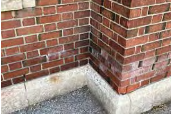
Fig. 1. Example of minimal spalling and efflorescence.
