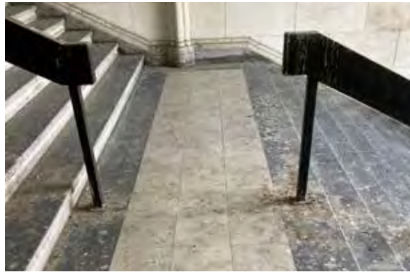
Fig. 37. Soiling at base and floor.
