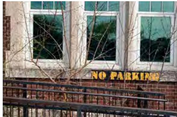
Fig. 19. Example of overpainting on exterior sills.
