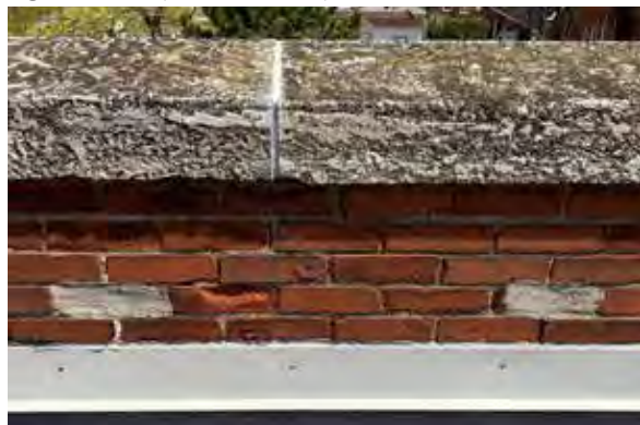
Fig. 76. Incompatible brick replacements.
