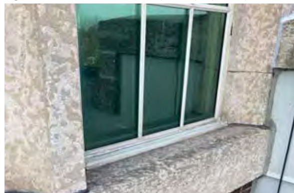
Fig. 33. Washed out joints are visible behind growth.
