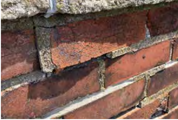
Fig. 70. Brick and mortar failure underneath parapet stone.
