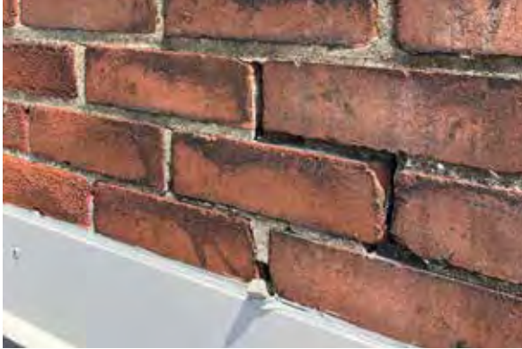
Fig. 71. Significant lose of mortar joints.
