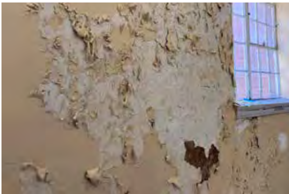
Fig. 104. Moisture damage to plaster and paint.
