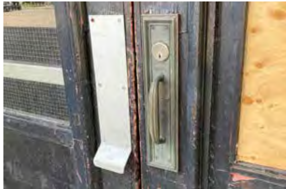
Fig. 88. One original handset and one replaced push plate.
