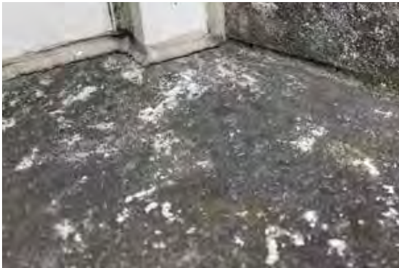
Fig. 40. Debonding between stone and caulking.
