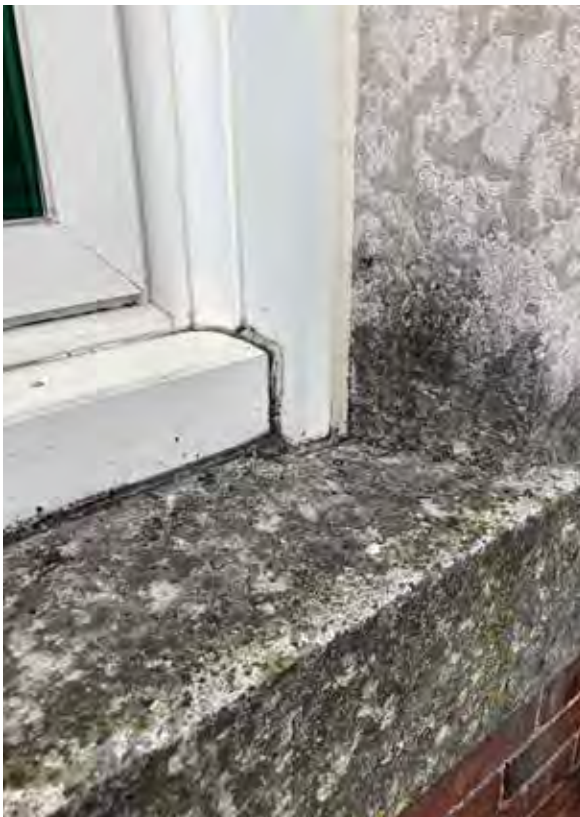
Fig. 17. Significant stone staining and organic growth.
