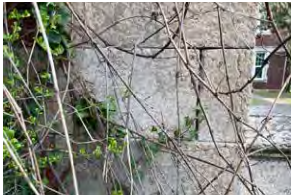
Fig. 29. Washed out joints are visible behind growth.
