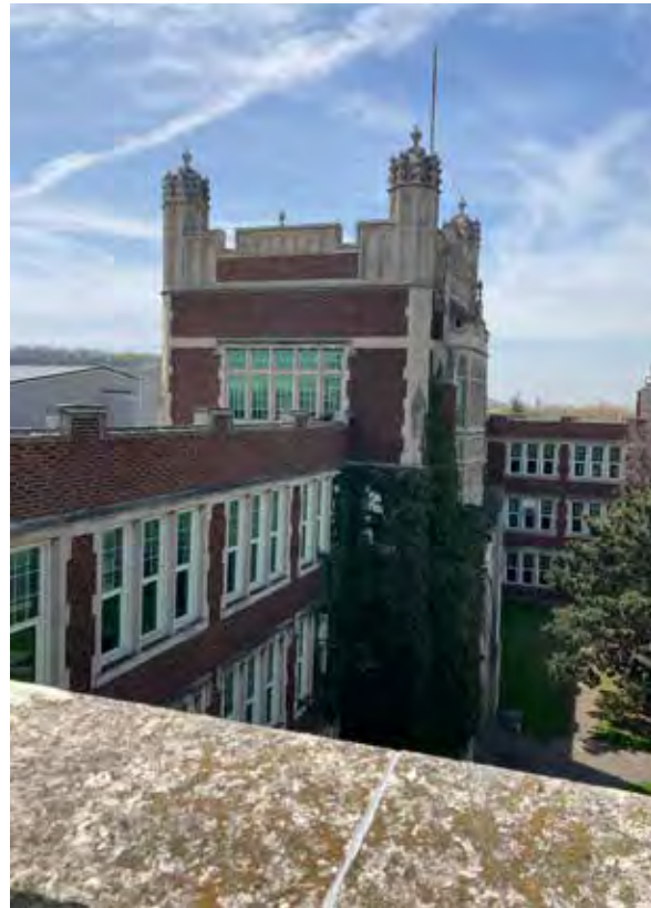
Fig. 31. Evidence of patch repair damage to stone.
