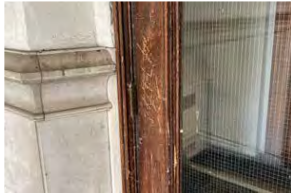
Fig. 78. Surface scratching of northern entrance door.
