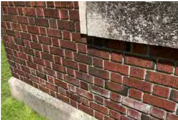
Fig. 3. Example of efflorescence towards base of exterior.
