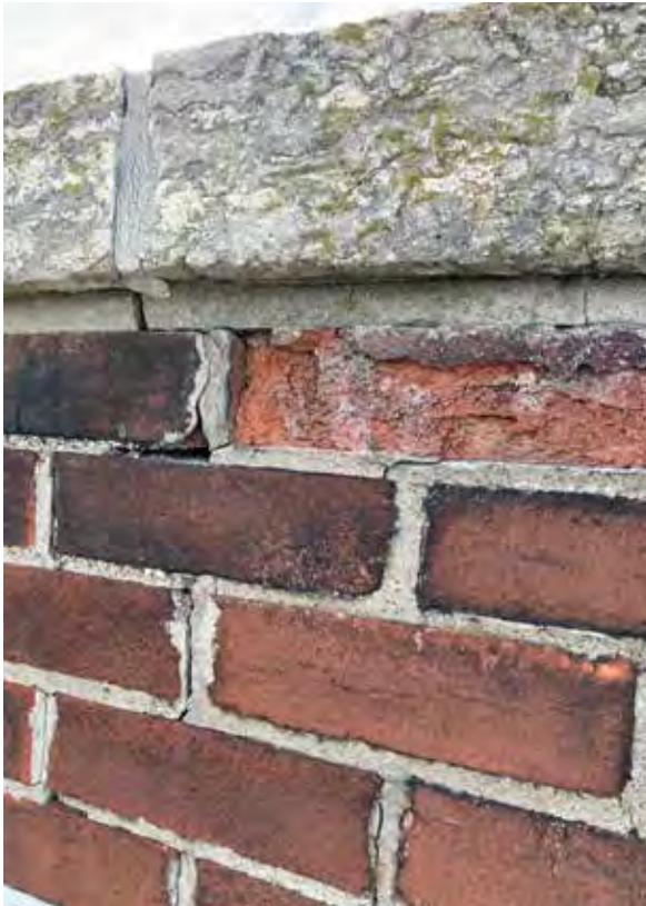
Fig. 72. Mortar cracking between bricks.
