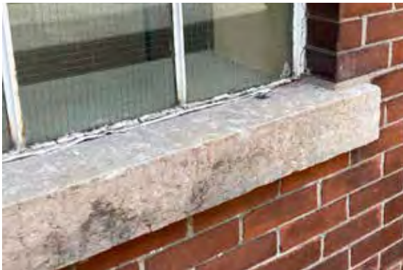
Fig. 58. Failed caulking joints at window sills.
