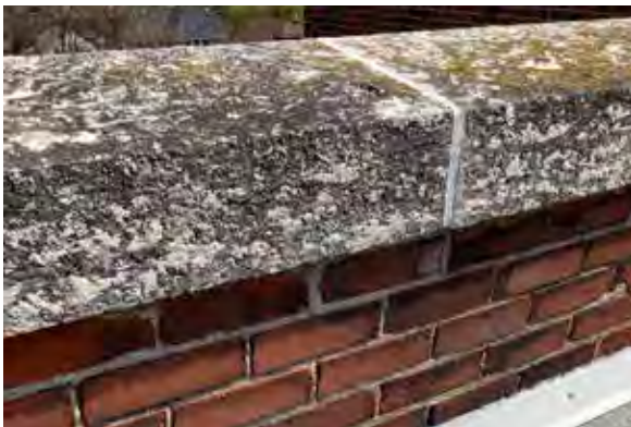
Fig. 65. Area of stone degradation.
