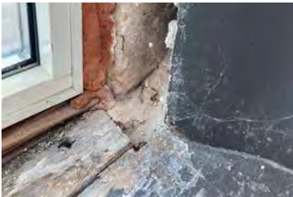
Fig. 109. Failed concrete sill.
