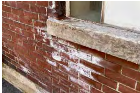
Fig. 48. Severe efflorescence and some spalling.
