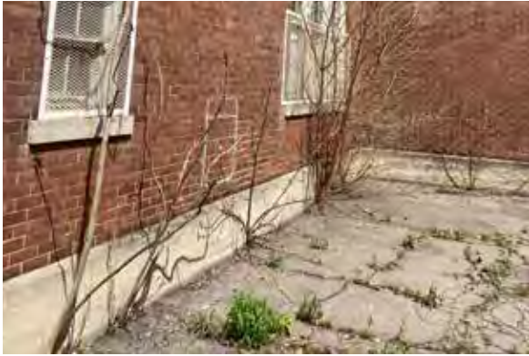
Fig. 52. Vegetal growth at base of north wall.
