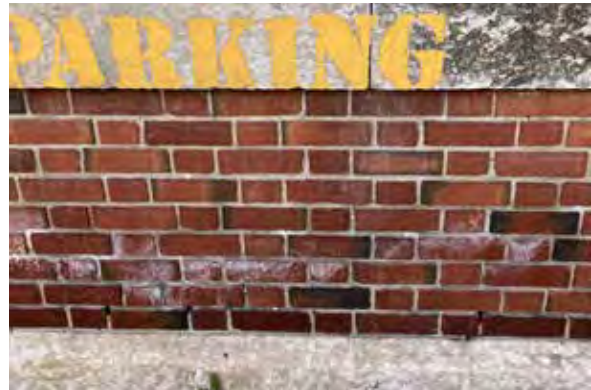
Fig. 7. Example of efflorescence towards base of exterior.
