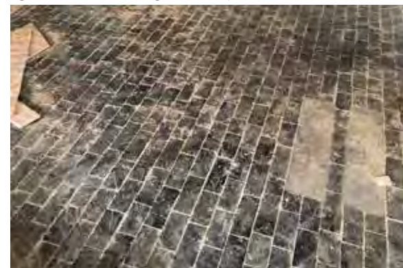
Fig. 117. Block flooring concrete patches.
