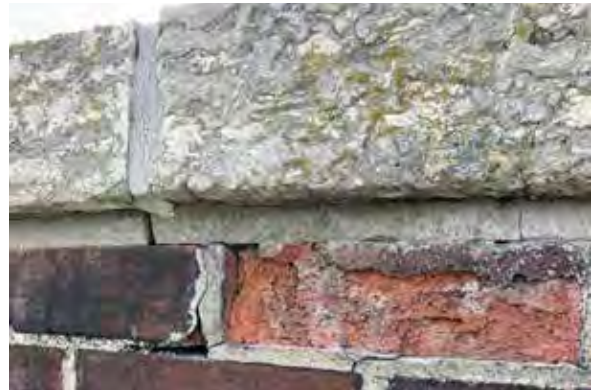
Fig. 61. Failed mortar joint.
