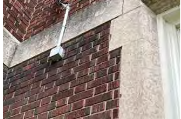
Fig. 13. Areas of minor stone chipping surrounding window.
