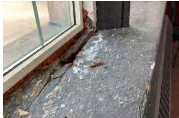
Fig. 112. Deteriorated wooden sills.
