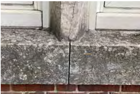
Fig. 12. Example of stone cracking.
