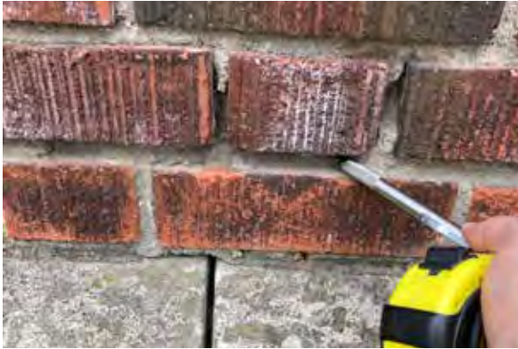
Fig. 10. Recessed mortar joints.
