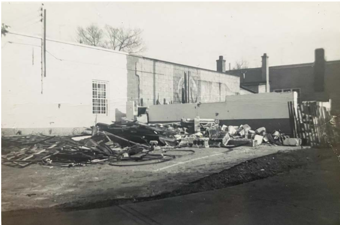
PATON MOTORS – the Texaco Service Station demolition complete – the garage building remains
