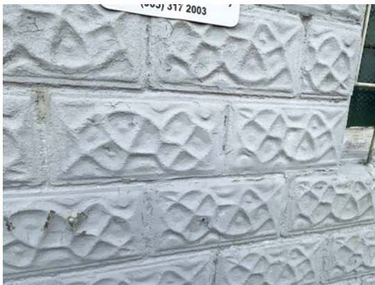
PATON MOTORS – EXTERIOR – side elevation facing King Street West – textured concrete block & wood sash windows
