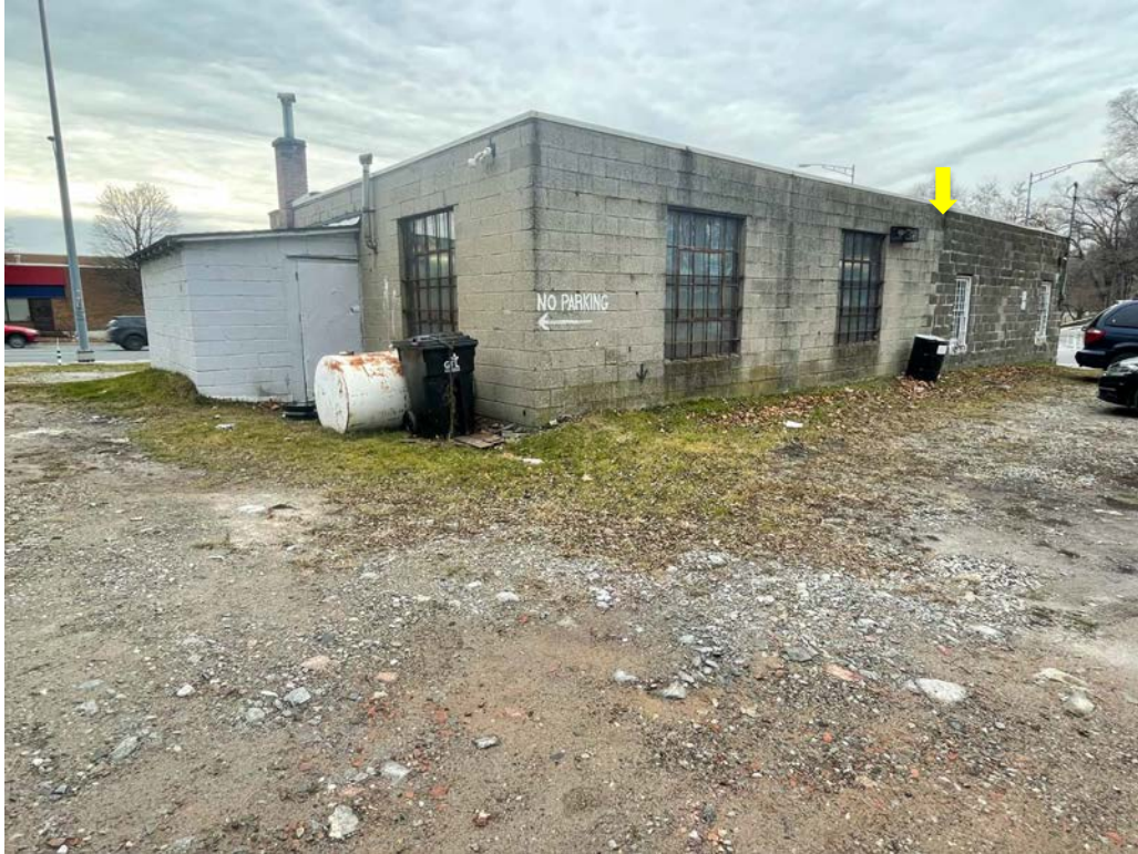
PATON MOTORS – EXTERIOR – rear and north side elevation – built in two phases: the concrete block & steell window portion at the East end (2 bays) was an extension to the earlier cinder block & wood window garage (2 bays)
