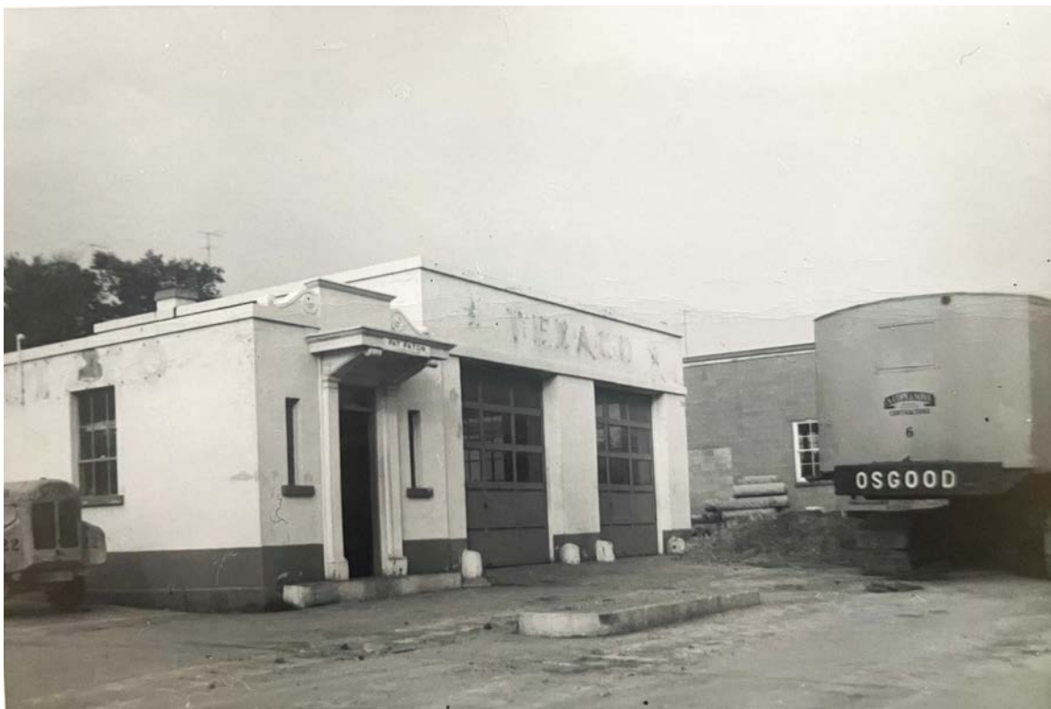
PATON MOTORS – Texaco Service Station demolition begins - the gas pumps & Texaco Sign have been removed
