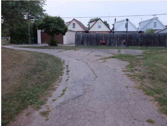
Figure 5: Pavements have reached the end of their service life (location Weir and Tragina trail segment), OMC photo
