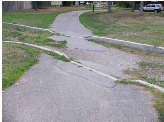
Figure 4: Existing paving conditions do not meet current accessibility requirements, OMC photo
