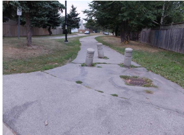
Figure 6: Example of bollards requiring replacement (location Fairfield to Paling trail segment), OMC photo
