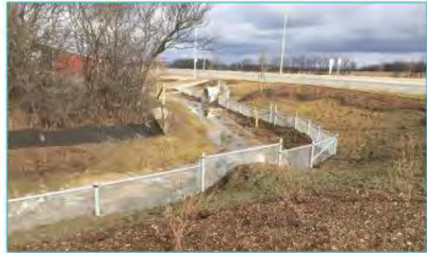
Wildlife Fencing, Tremaine Rd, Milton, Ontario
