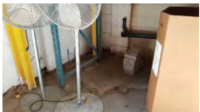
Photo 24 – View of the former paint mixing room inside the 2 Hillyard St building. Staining was observed on the concrete floor where the former solvent tanks would have been located.
