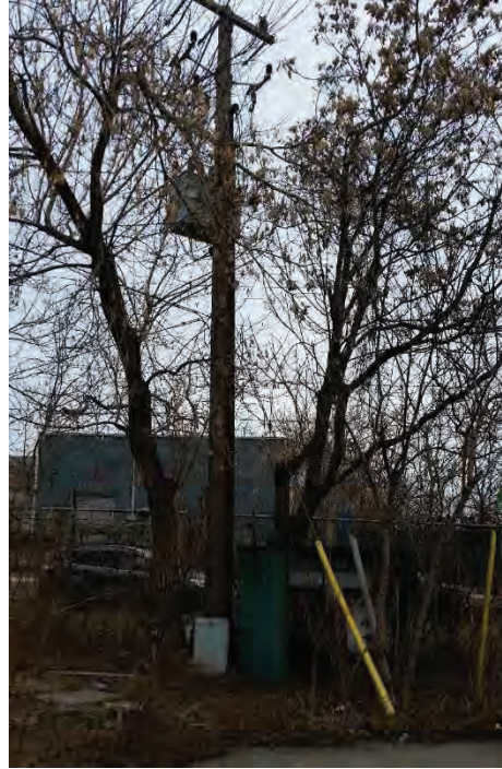
Figure 3-5 Photo showing overhead power supply and transformer cabinet
