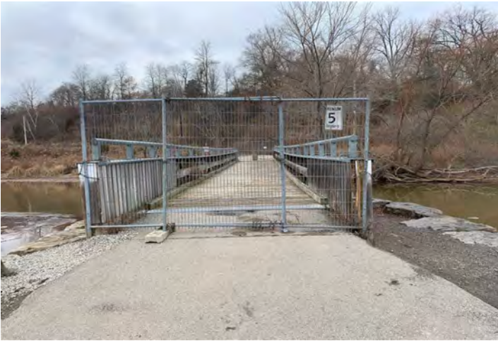
Photo 1: Facing west towards Valley Inn Bridge from east end of the bridge.
