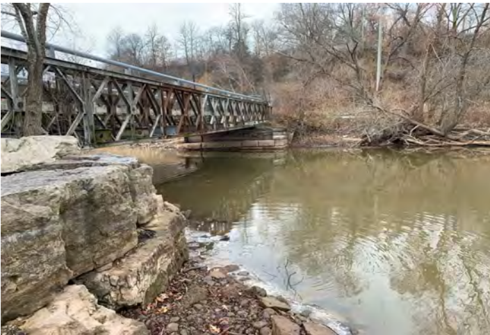
Photo 5: Upstream side of the Valley Inn Bridge, facing the west shoreline and abutment.
