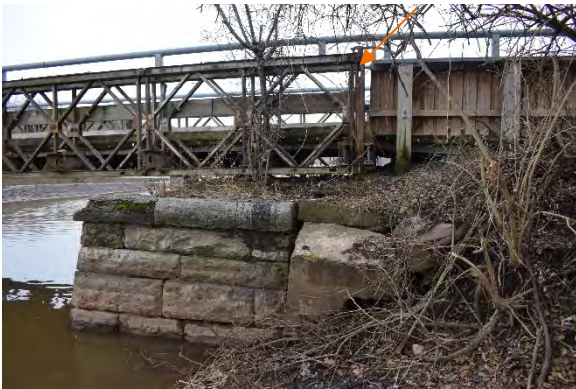
Plate 21: Stone abutment and original southwest end post (denoted by arrow), looking south
