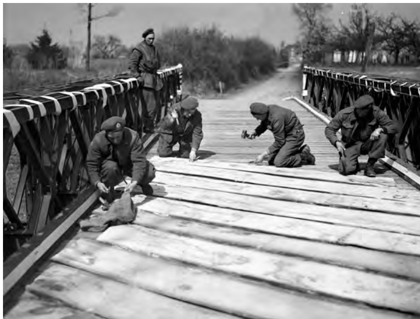
Plate 27: Personnel of the 18 th Field Company, Royal Canadian Engineers, constructing a Bailey Truss Bridge in the Netherlands in 1945 (Library and Archives Canada 1945)
