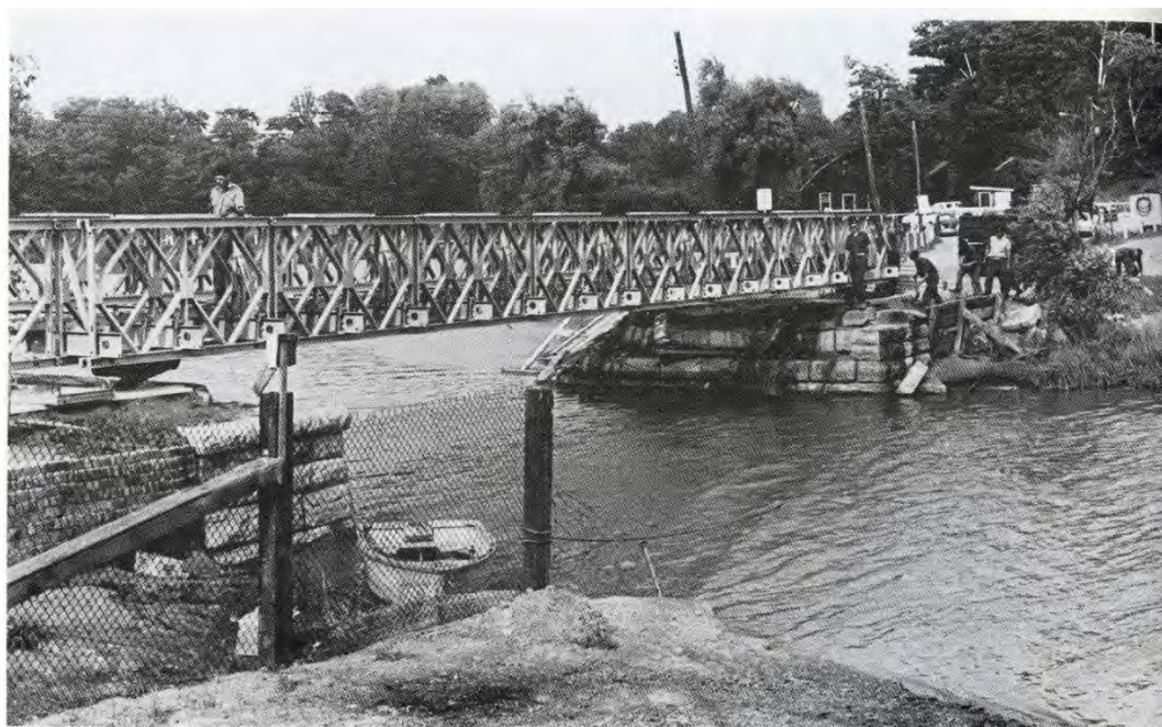
Plate 25: The 47 th Field Squadron of Royal Canadian Engineers installing the Valley Inn Bridge in 1964(Evans 2000)
