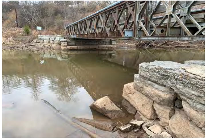
Photo 2: Downstream side of the Valley Inn Bridge, facing west from the east abutment.
