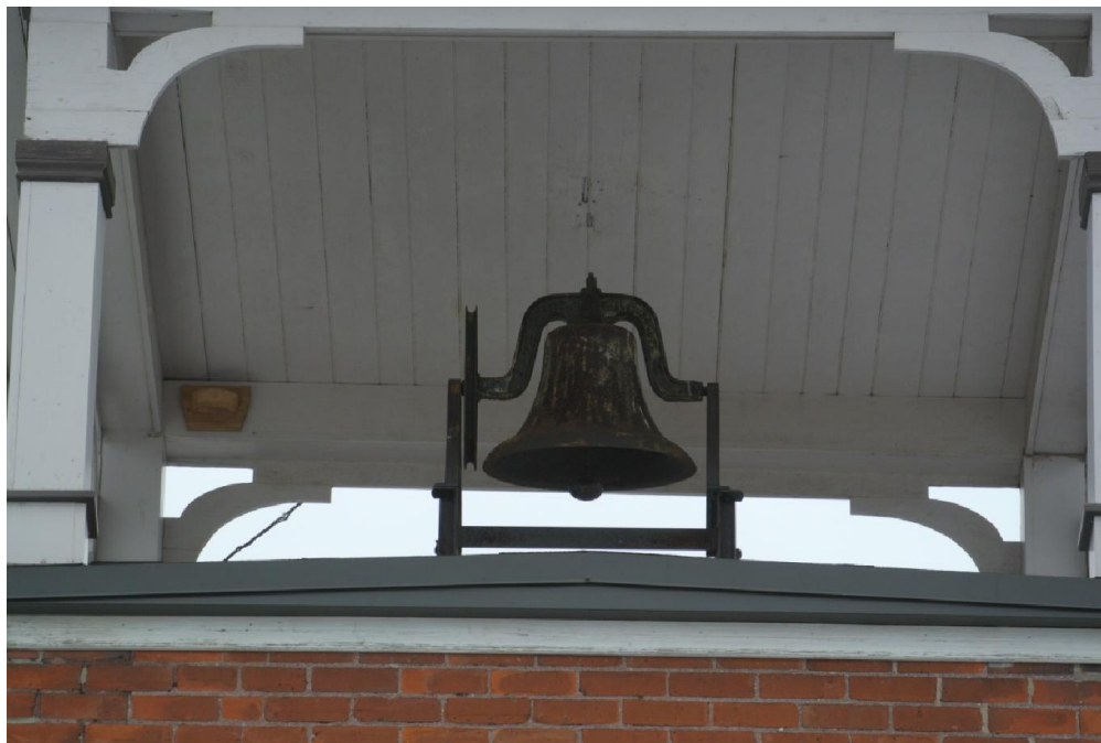
Plate 8: Detail of the bell and wood slat soffit of the bell tower.
