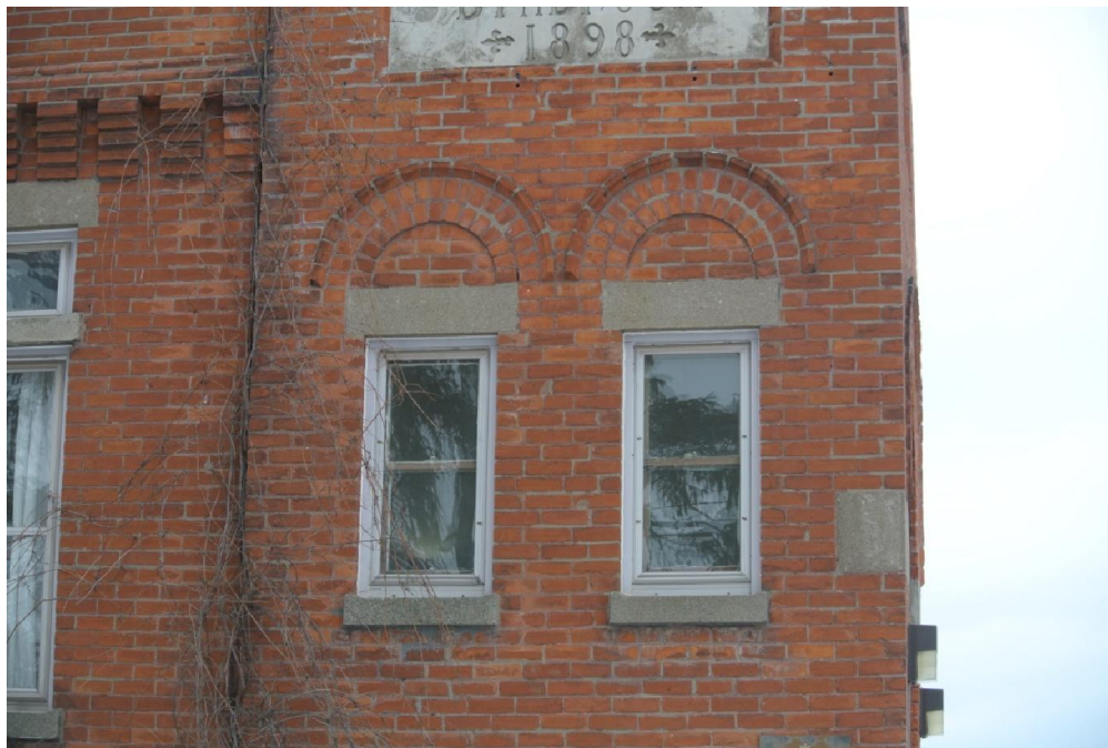
Plate 12: Detail of the fenestration on the south elevation of the bell tower.
