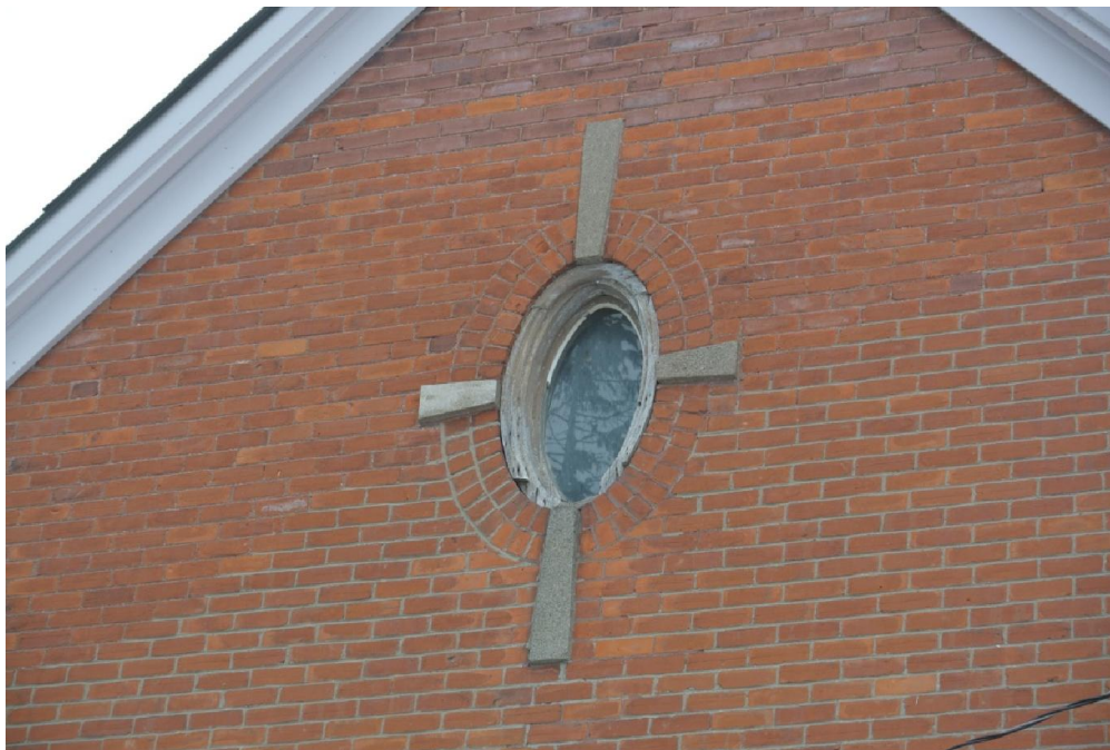
Plate 14: Detail of the oval window in the gable end of the south elevation.
