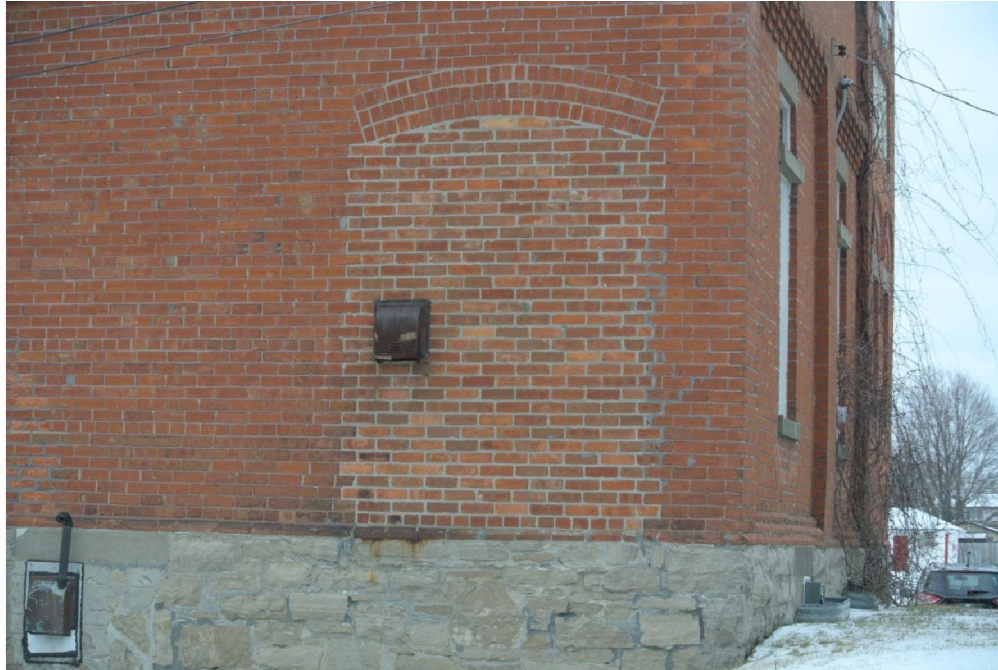
Plate 15: Detail of the former opening that has been bricked in on the west elevation.
