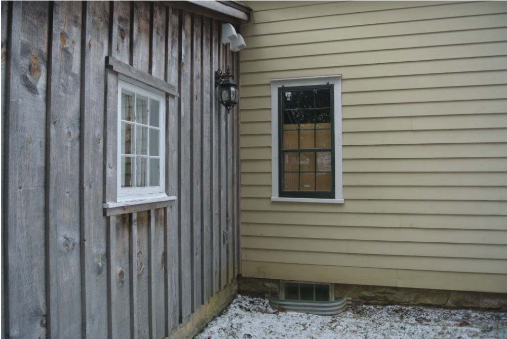
Plate 10: View toward the east elevation. Note the board-and-batten siding of the modern addition.
