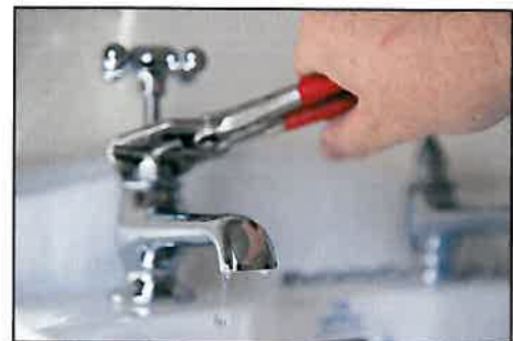
Leak Detection and Elimination (Source Farmers' Almanac)
