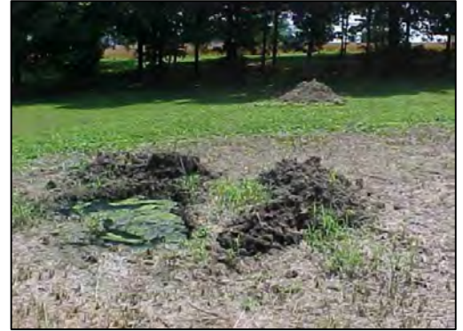
Failed Septic System (Source ORWC)
