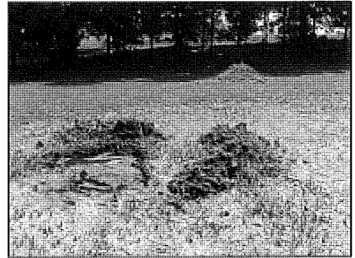
Failed Septic System (Source ORWC)
