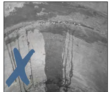
A leaky cement casing could lead to contamination. (Source WellAware.ca)
