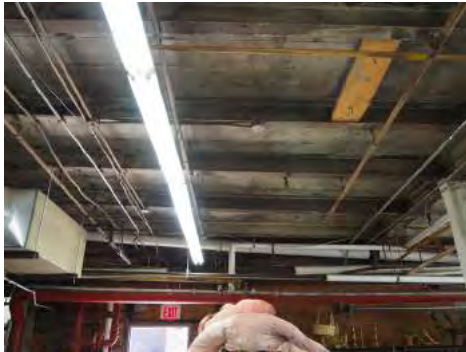
Exposed concrete ceiling (functioned as a 'wet floor' on Level 2) and steel beams.
