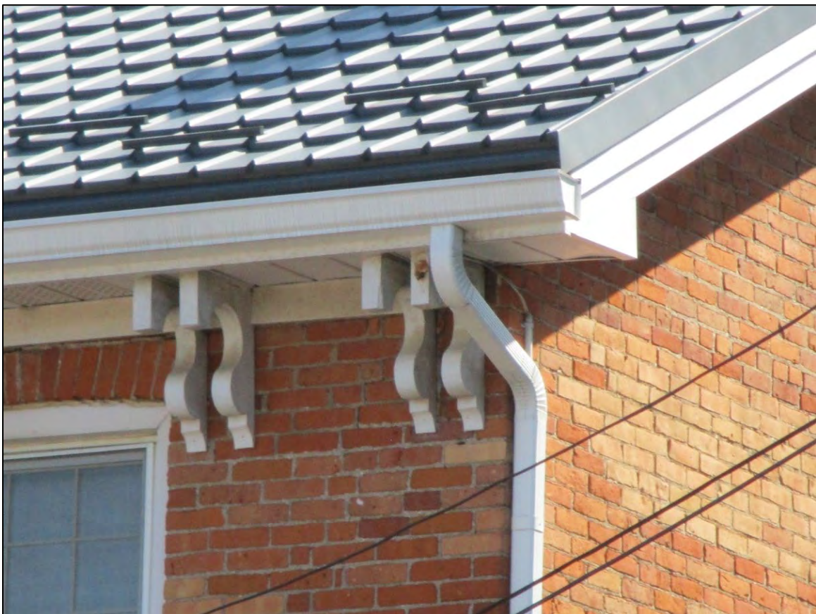
Image 10: Detail of brackets on western end of the north elevation of the rear wing.
