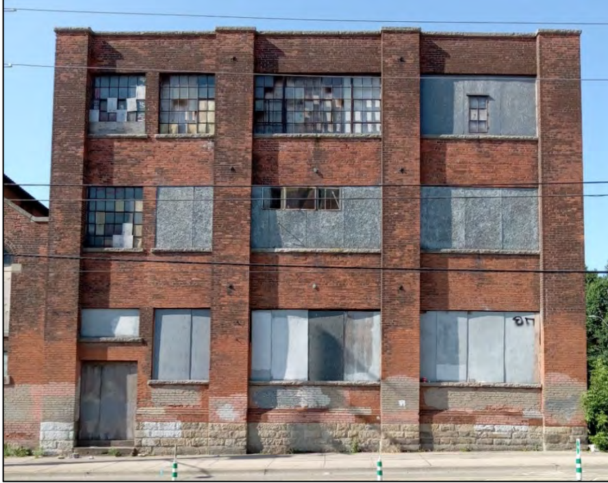
Figure 7: View of the north façade of the western portion of 140-146 Mary Street (Structure 4) facing onto Cannon Street East.
