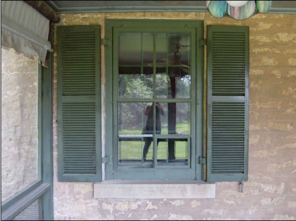
Figure 11: Detail view of window on south elevation showing wooden storms and shutters and stone sill.
