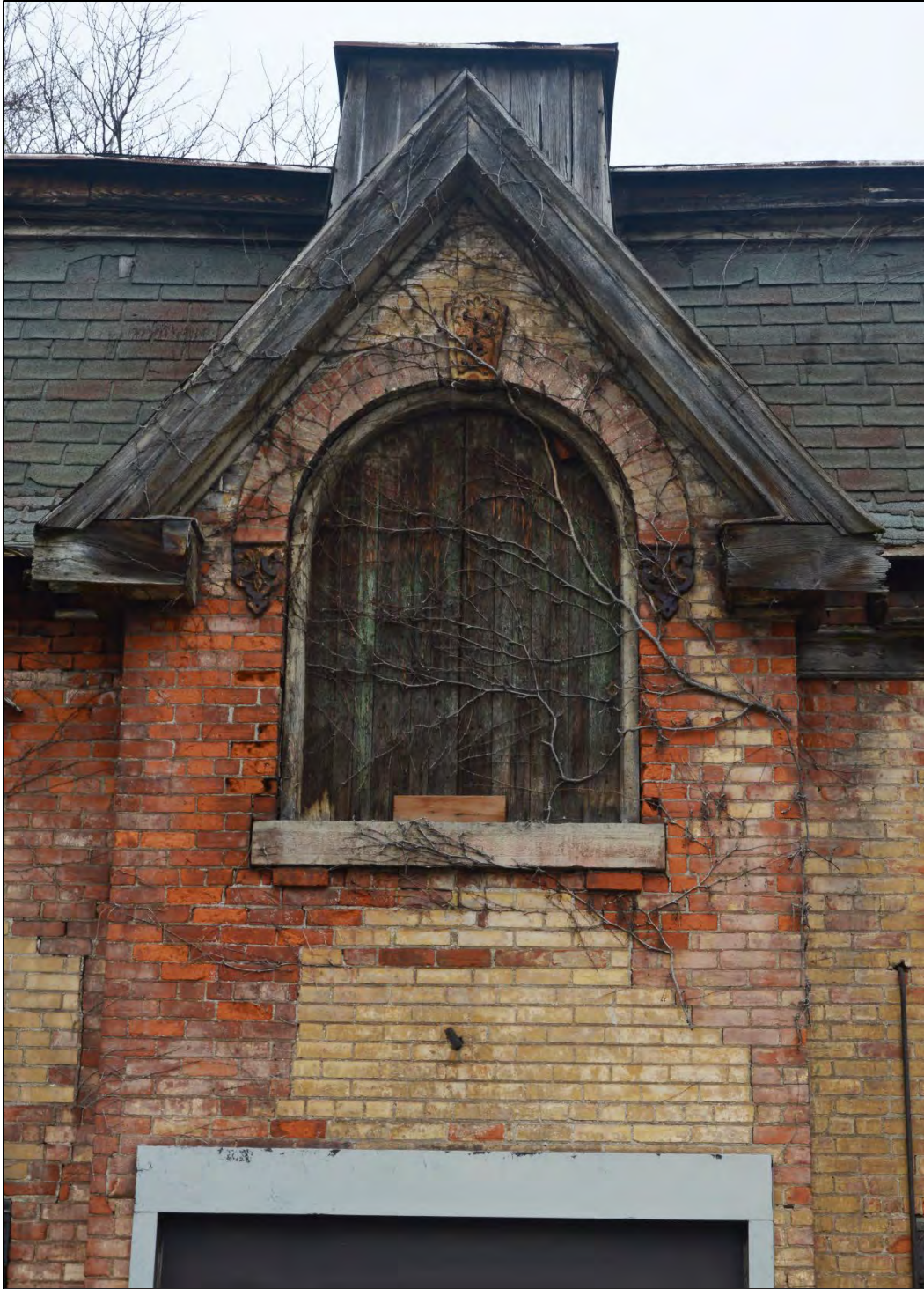
Image 14: Image of the second storey window opening on the southern elevation. Note the rust on the cast iron ornaments. Image by Graham Carrol and Ann Gillespie, 2019.
