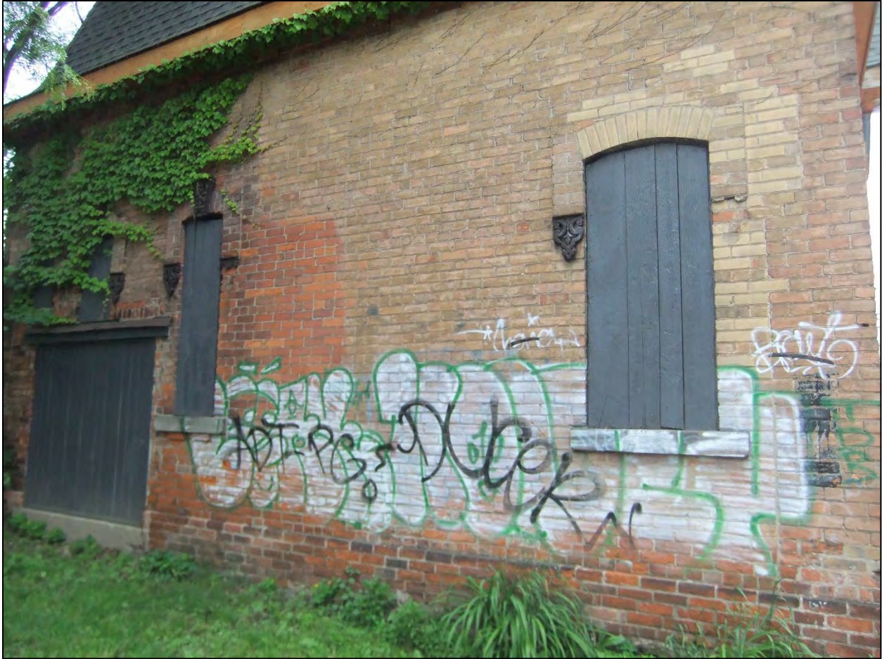
Image 6: Western elevation, take note of the truncated door and window openings on the left-hand side of the image.
