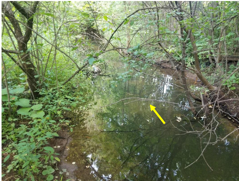
Evidence of erosion largely subsides near the downstream extent, as the channel exhibits more depositional tendencies, indicated by siltation on the bed.
