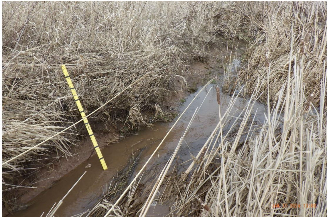
Basal scouring was observed throughout the reach, in particular at the downstream section. Bed and bank materials consisted primarily of clay.
