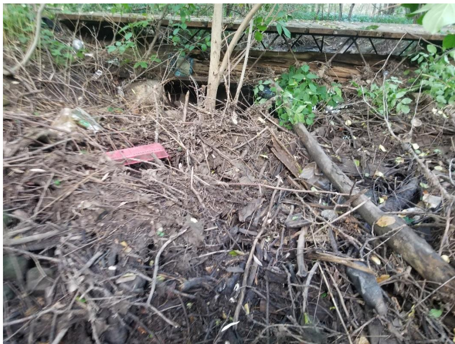
A small footbridge is present in WC5 . A thick debris jam exists immediately upstream and retains a level of flow.
