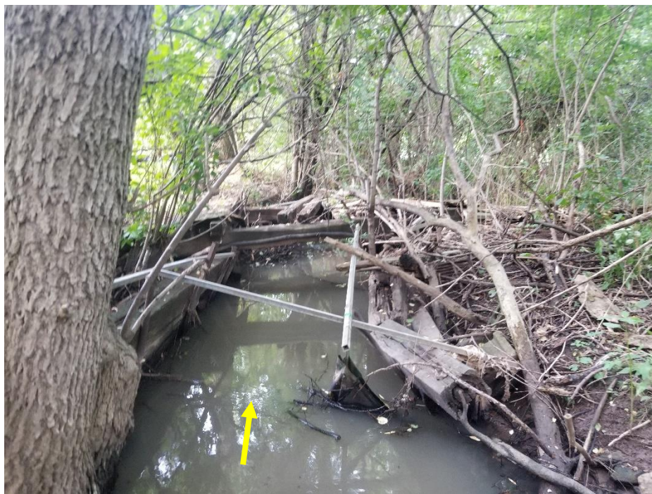
Bank armoring and a footbridge were observed further downstream. This infrastructure is significantly degraded and has evidently not been maintained for many years.
