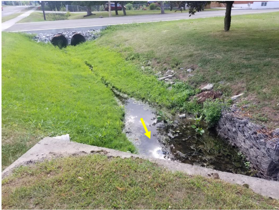
Flows enter reach WC5 through a concrete box culvert passing under Fruitland Road. No erosion concerns were noted. Yellow arrow denotes flow direction.
