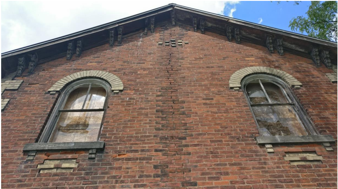
Figure 20.0: Large Gaps in Brick Joints on East Face
