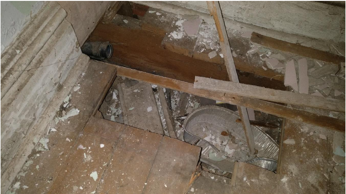
Figure 10.0: Typical Existing Floor Joists on 2 nd Floor 2"x10" timber floor joists at 18" o/c with 1" wood T&G decking
