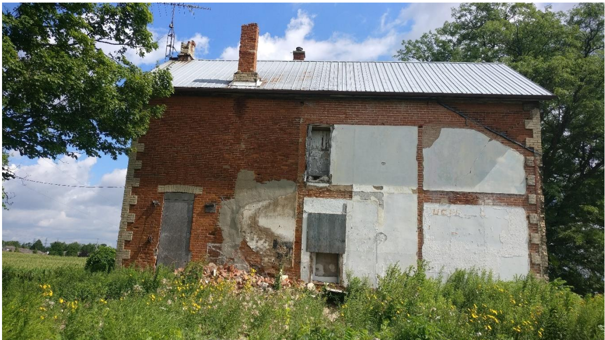
Figure 6.0: South Façade of Building Evidence of south addition with parged and discoloured brick
