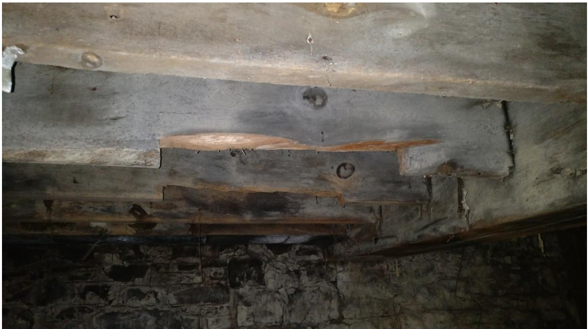
Figure 12.0: Multiple Notched Ground Level Floor Joists Floor joists supported by large wood beam on right side
