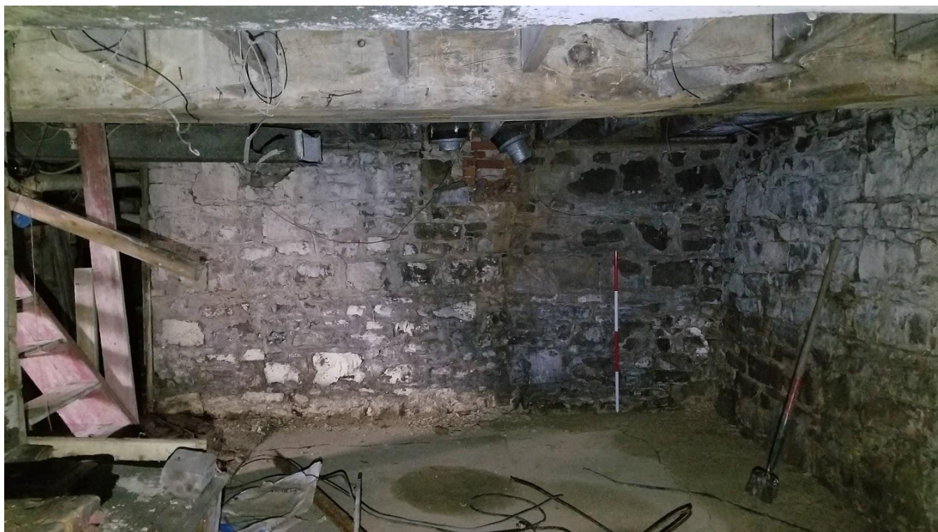
Figure 113: 9285 Twenty Road West: Room with exposed wood joists, stone walls and hand hewed beam
