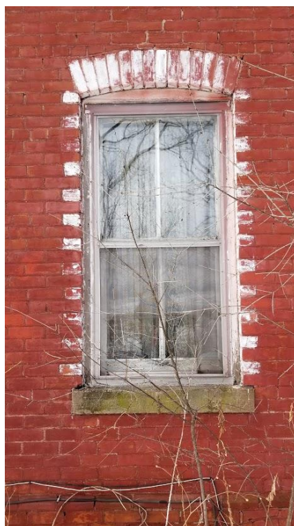
Figure 41: 9751 Twenty Road West: Segmental arch window with soldier brick voussoirs painted white and bush hammered lug sill
