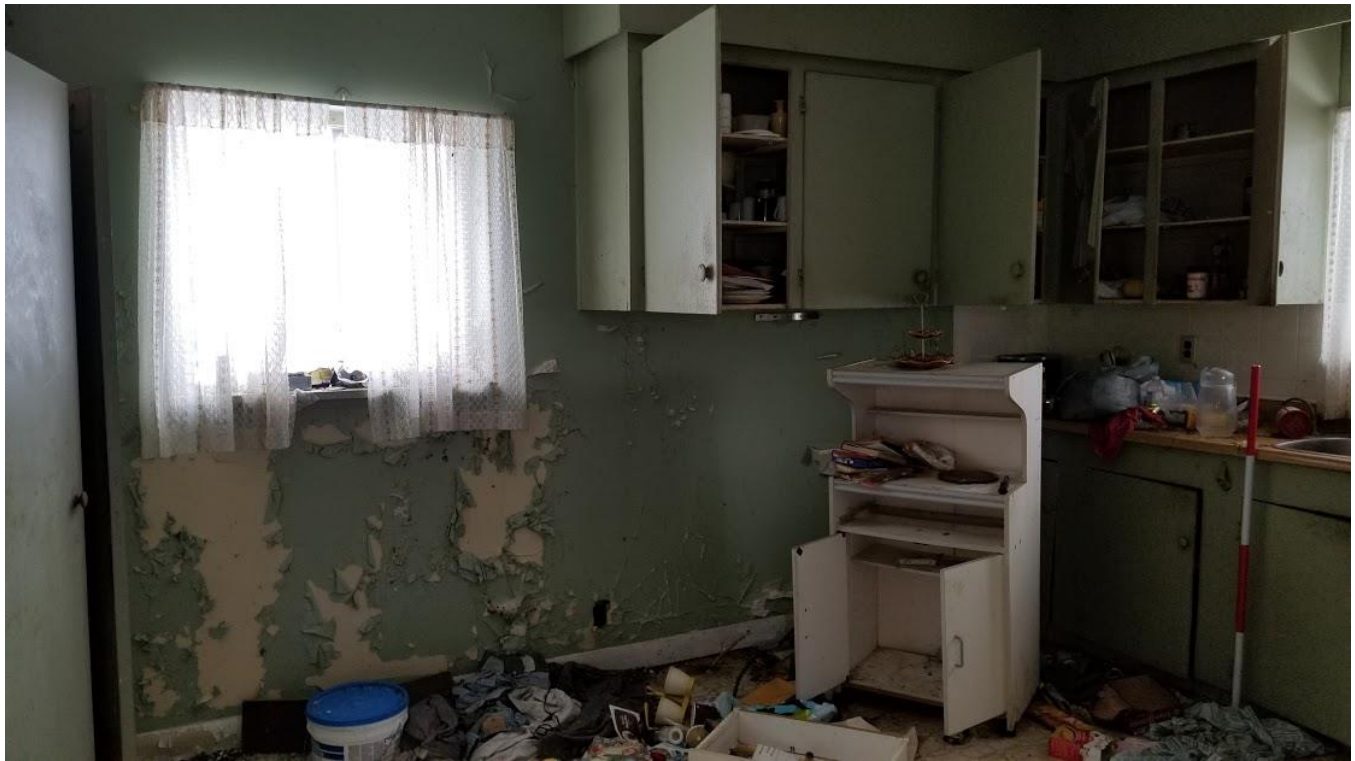
Figure 53: 9751 Twenty Road West: Former kitchen located at the northeast corner of the house
