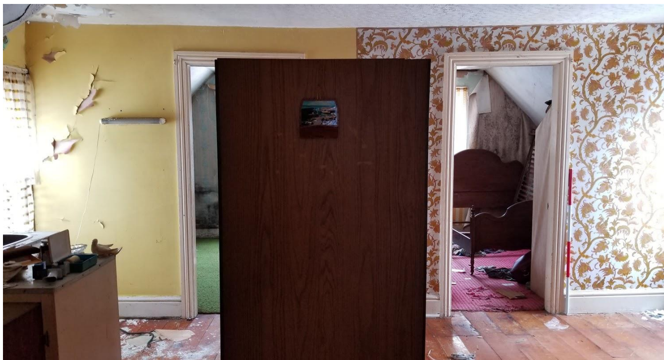
Figure 70: 9751 Twenty Road West: Large room to the north of the central hallway showing two additional rooms to the north
