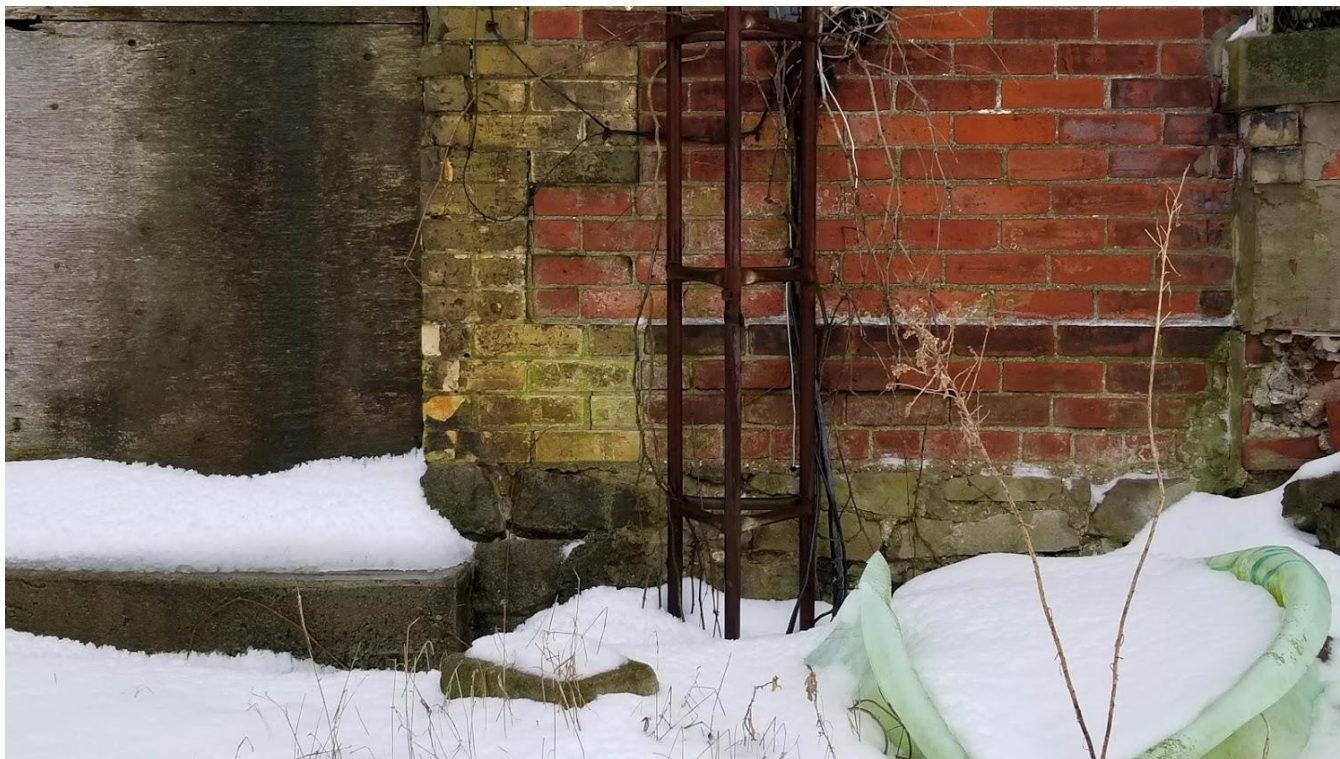
Figure 86: 9285 Twenty Road West: Coursed fieldstone foundation with stretcher brick, quoin detailing and water table
