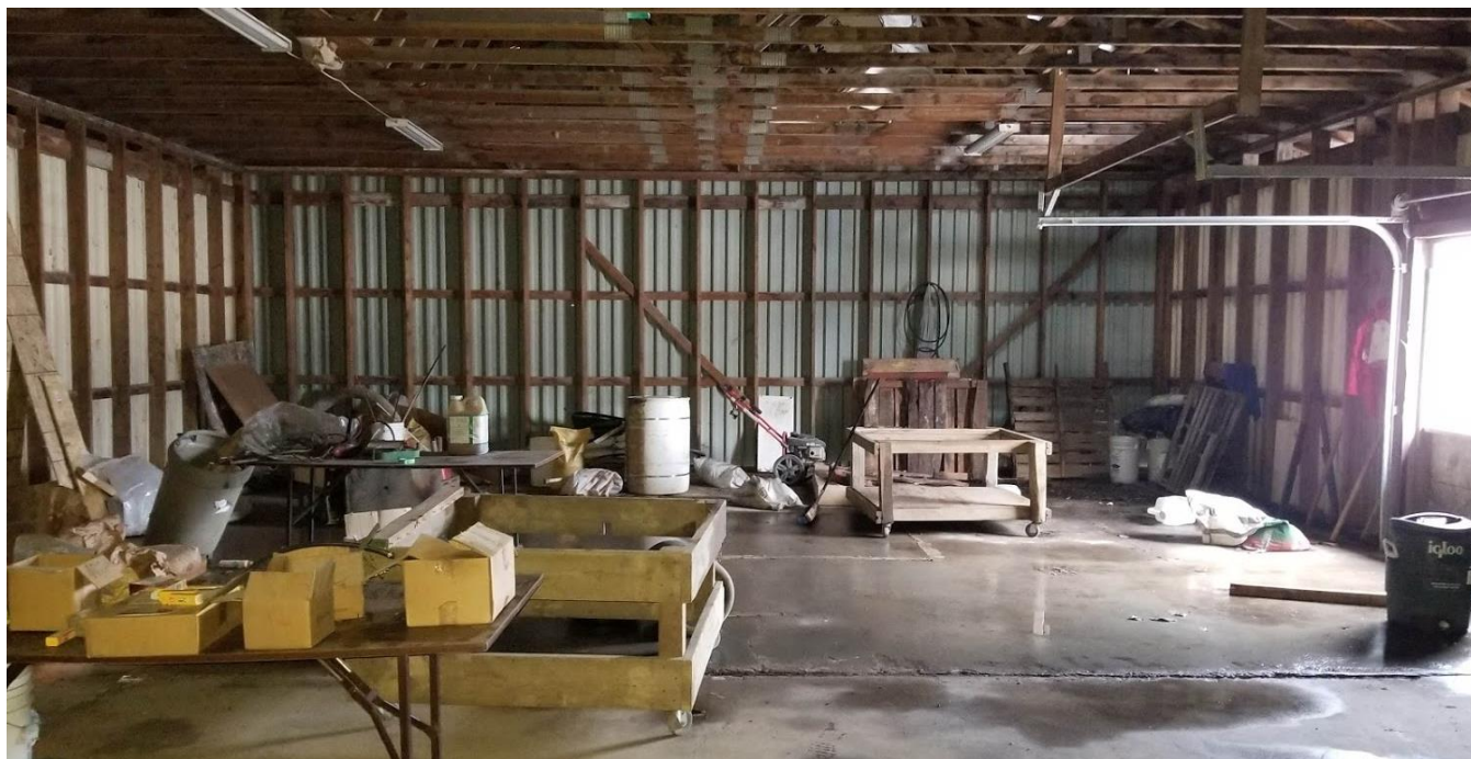
Figure 31: 555 Glanaster Road: Exposed light wood frame and roof trusses, with platform framing on the walls of the outbuilding
