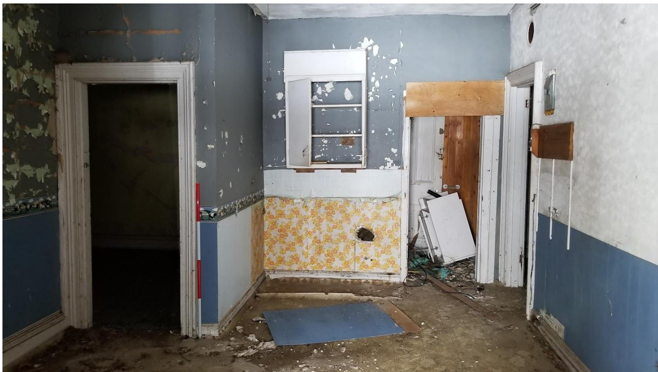
Figure 105: 9285 Twenty Road West: Second storey hallway providing access to a bedroom to the left and a washroom and bedroom to the right
