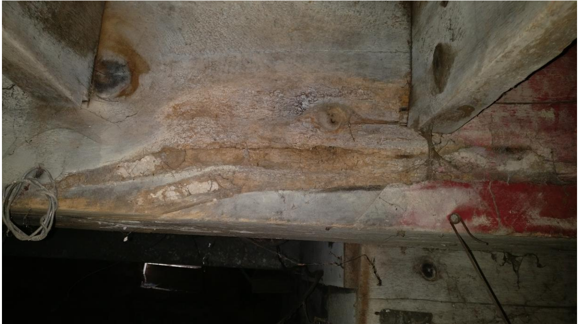
Figure 15.0: Termite Damage Noted on Large Wood Beam in Basement
