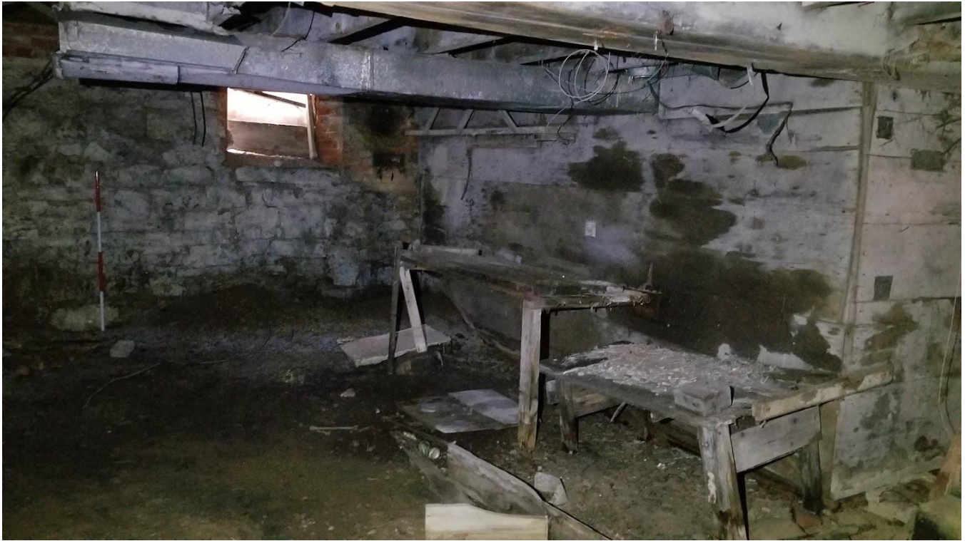
Figure 115: 9285 Twenty Road West: basement facing east with timber boards visible to the right
