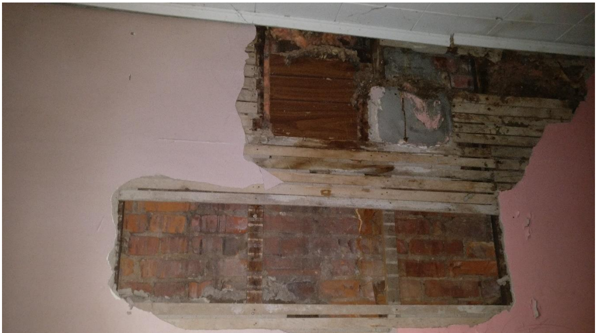
Figure 8.0: Interior Face of Exterior Brick Walls Multi-wythe brick with 1"x2" wood strapping, wood lath and plaster
