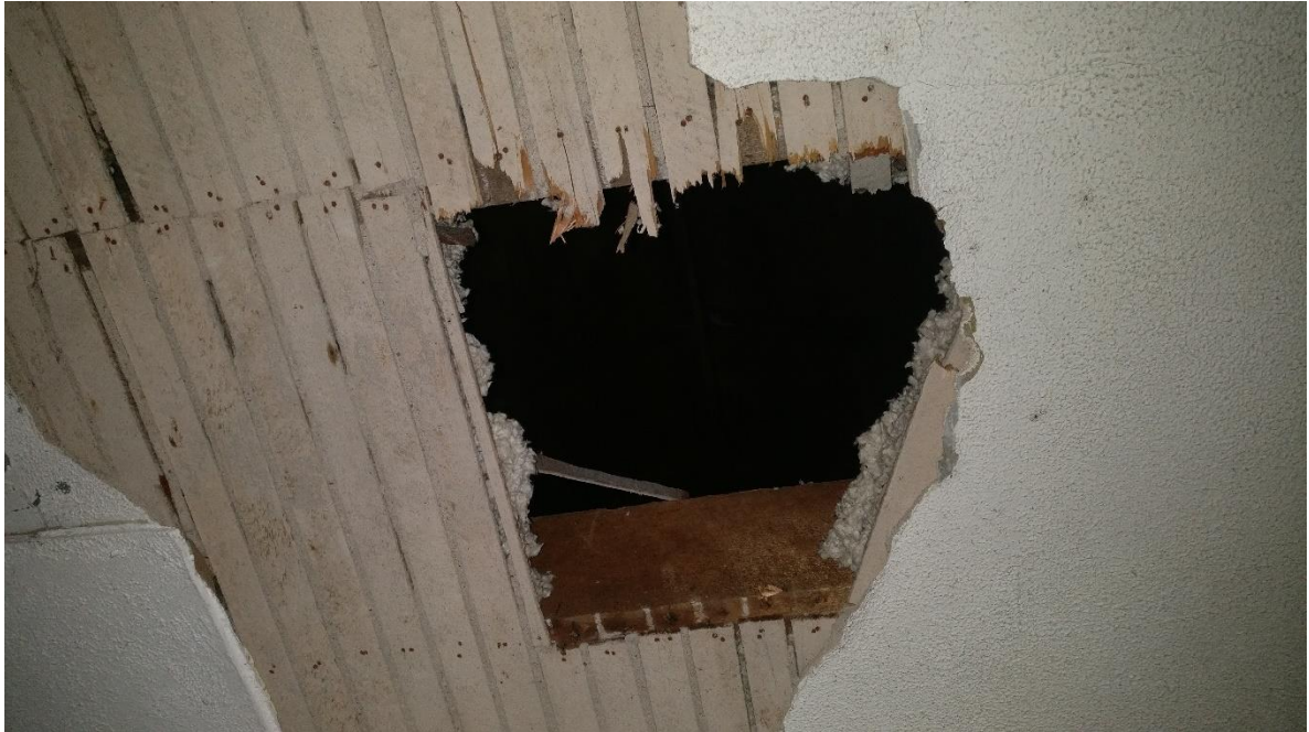
Figure 11.0: Typical Ceiling Wood lath and plaster on underside of ceiling and floor joists
