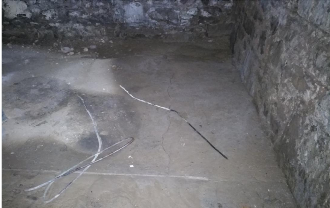
Figure 17.0: Small Portion of Slab on Grade in Basement Multiple cracks throughout slab Soil floor throughout majority of basement
