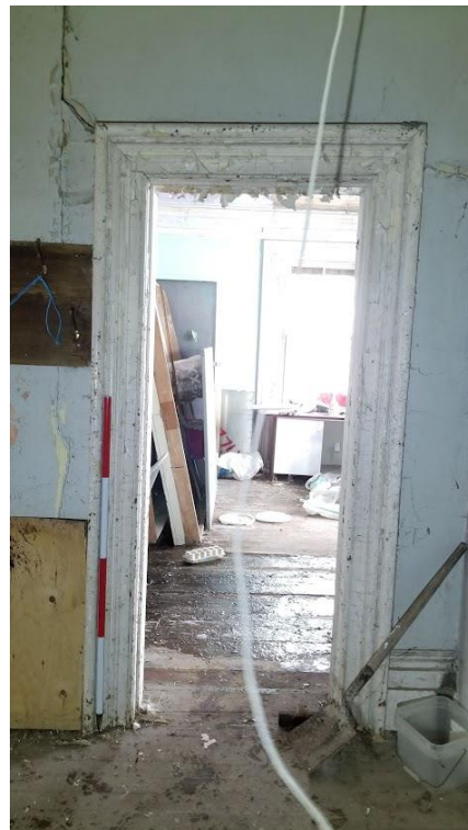
Figure 121: 9285 Twenty Road West: Water damage on the floors
