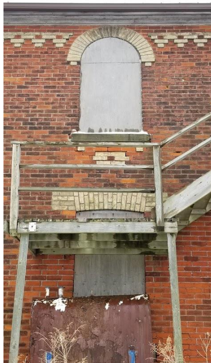
Figure 93: 9285 Twenty Road West: Main entrance on the first storey on the north façade
