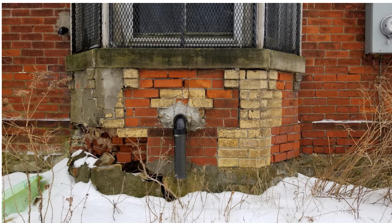
Figure 119: 9285 Twenty Road West: Missing brick at the corner of the bay window and evidence of concrete parging
