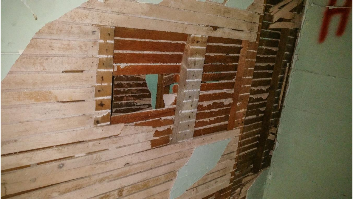
Figure 9.0: Interior 2 nd Floor Load-Bearing Wall 2"x4" studs at 18" o/c, rotated 90° with wood lath and plaster on each side
