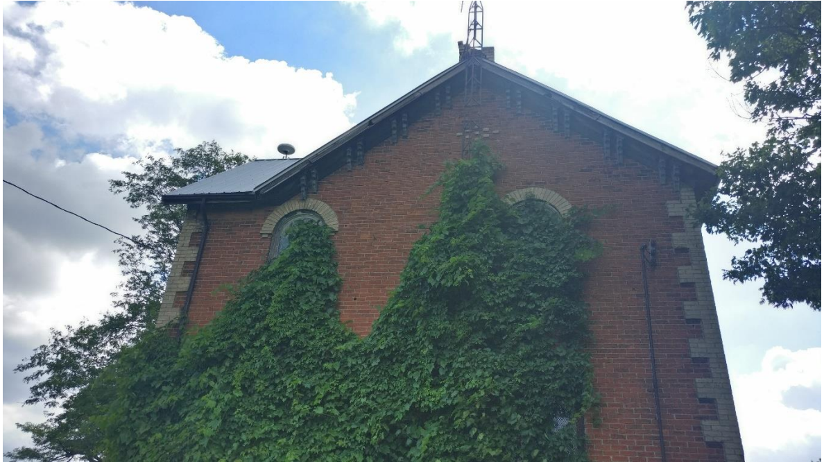
Figure 7.0: West Façade of Building Vine growing up the face of the building hiding the condition of brick
