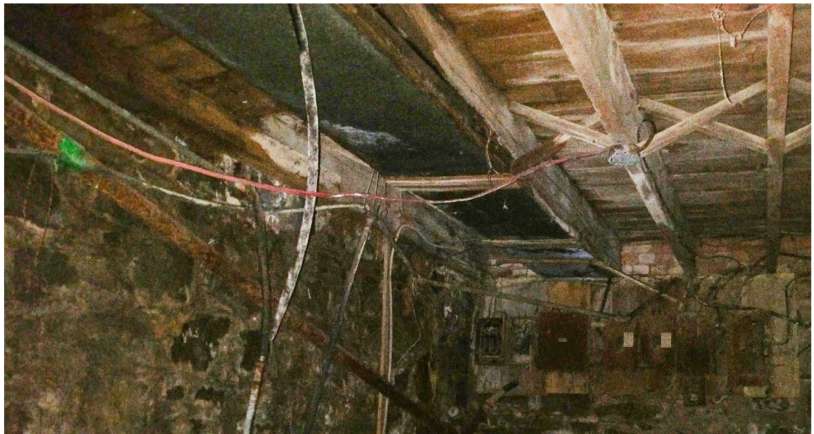
Figure 14.0: Existing Ground Level Floor Joist at South-West Corner Significant water damage noted on floor joists and floor decking Floor joist second from left completely split apart
