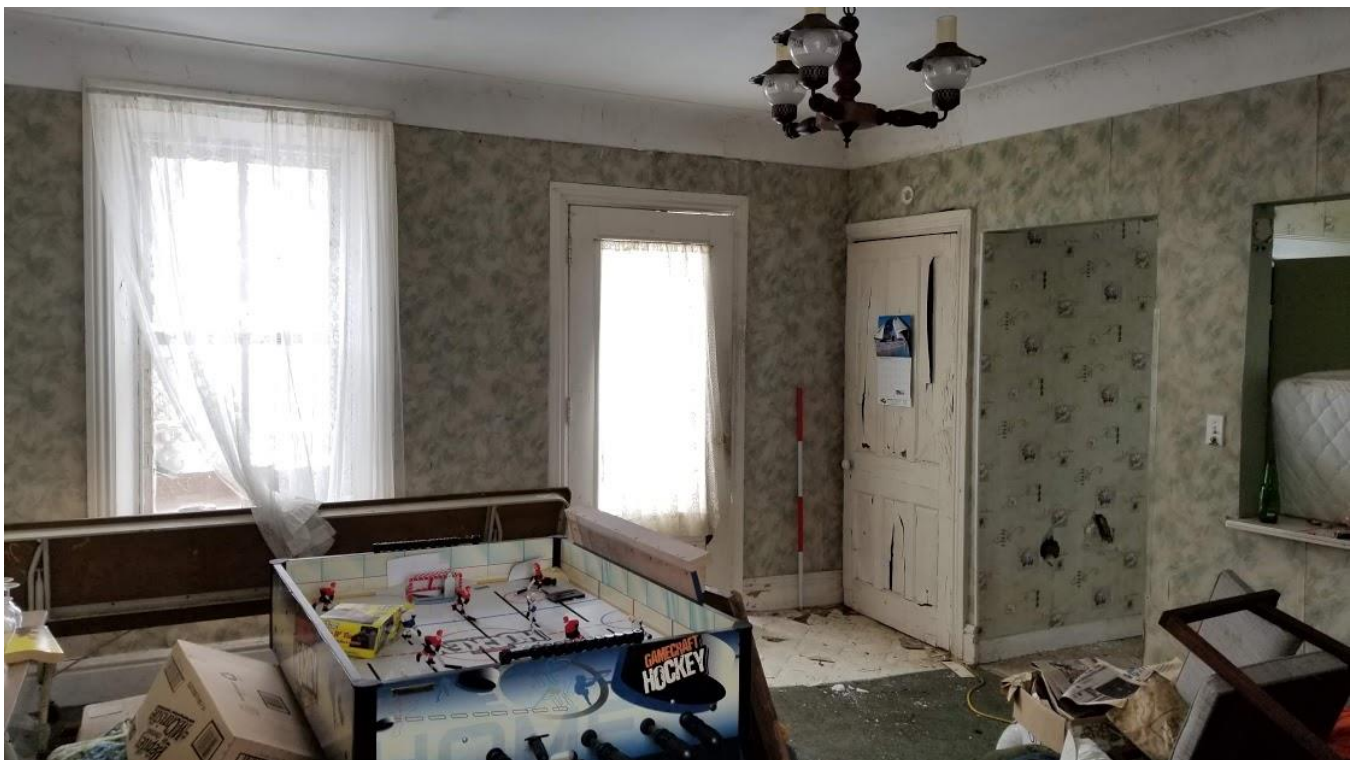
Figure 50: 9751 Twenty Road West: Main entrance on the west façade and wood door leading to the basement, and kitchen visible to the right
