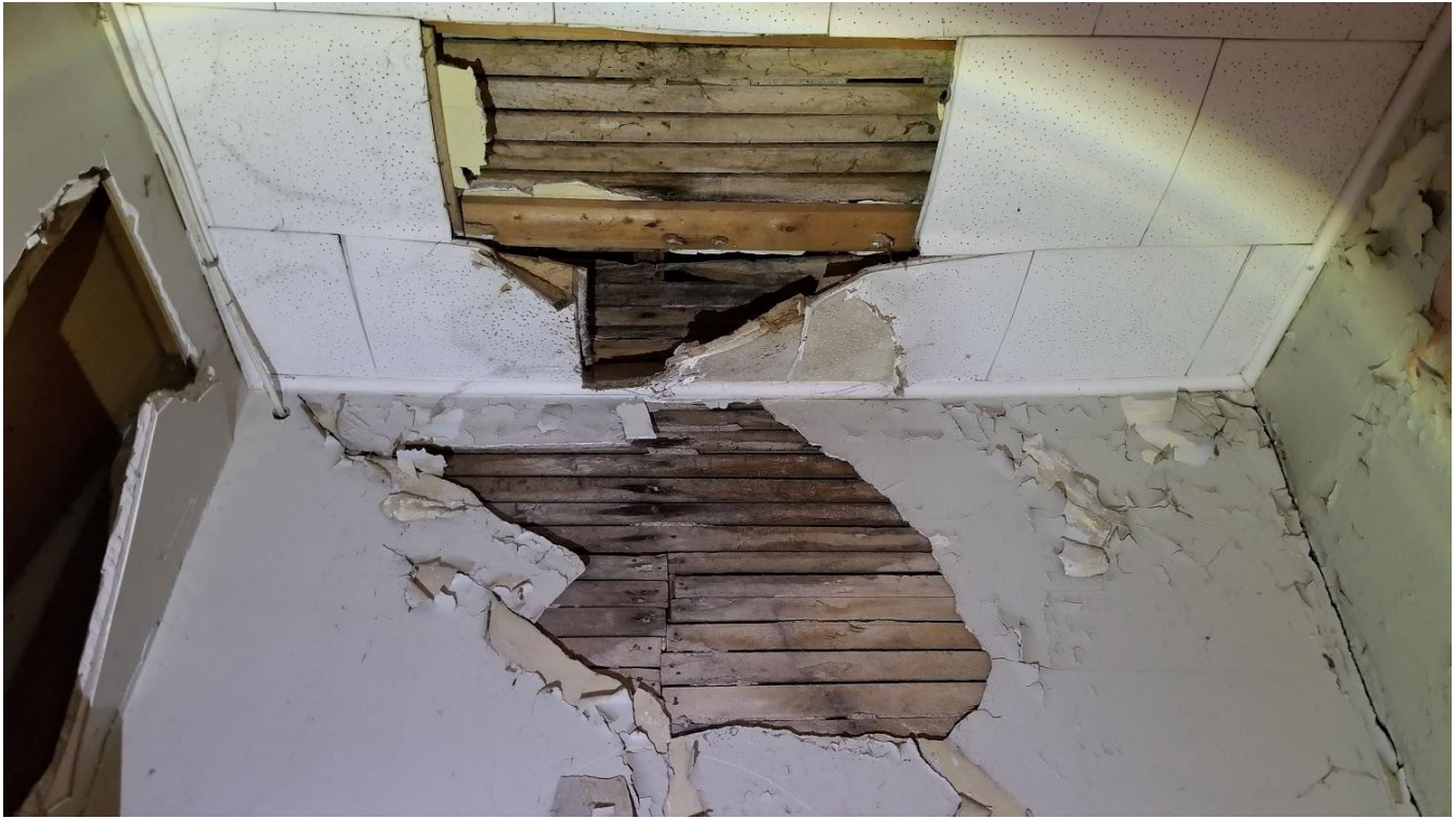
Figure 120: 9285 Twenty Road West: Exposed lathe from fallen plaster
