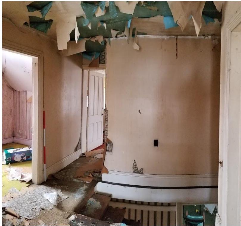
Figure 64: 9751 Twenty Road West: Central hallway facing north
