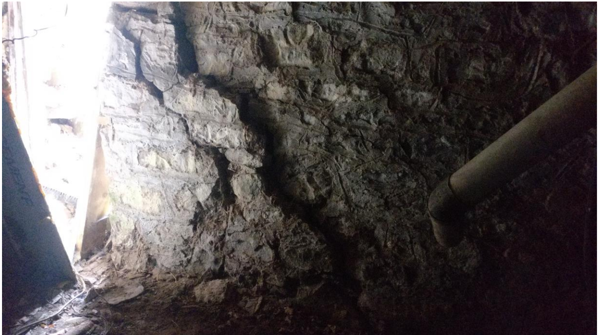
Figure 18.0: Severely Cracked and Shifted Foundation Wall
