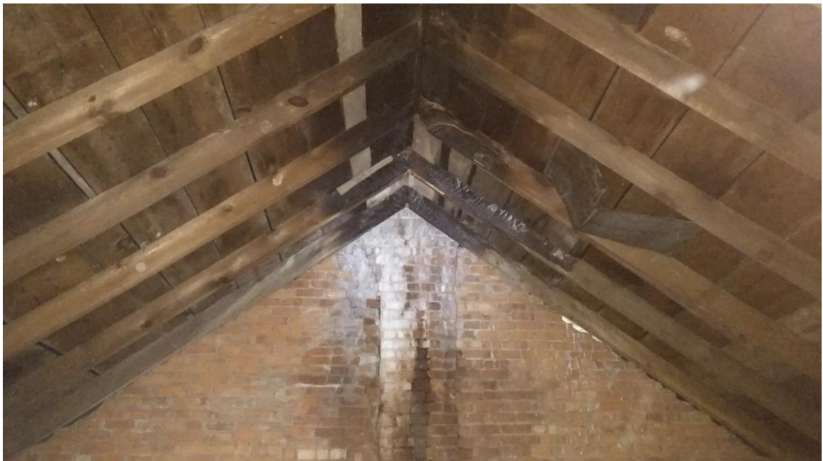
Figure 22.0: Roof Framing at East Side Rafters and planks charred showing evidence of fire damage
