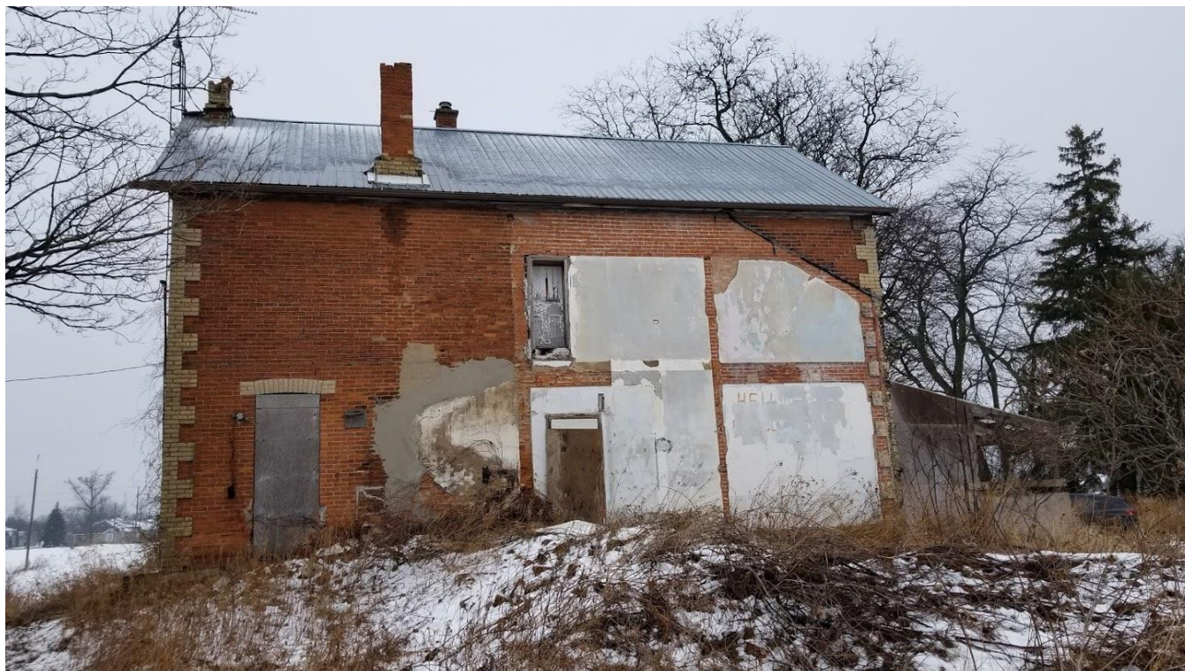
Figure 123: 9285 Twenty Road West: Concrete parging at the former location of the side-hall or gabled ell portion of the structure
