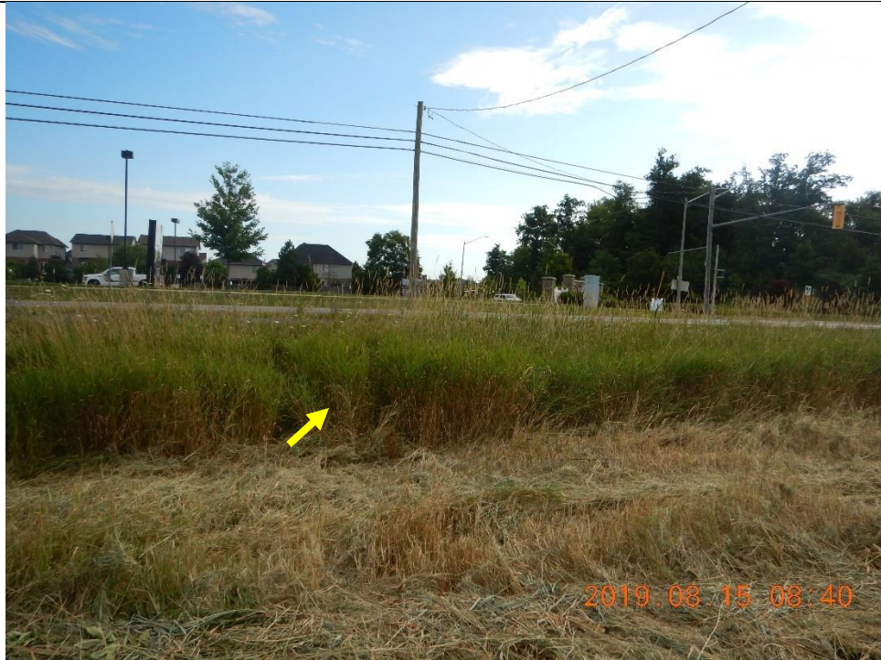
Bed material for the reach was predominantly clay, silt and sand. No water was present within the reach during the third visit.
