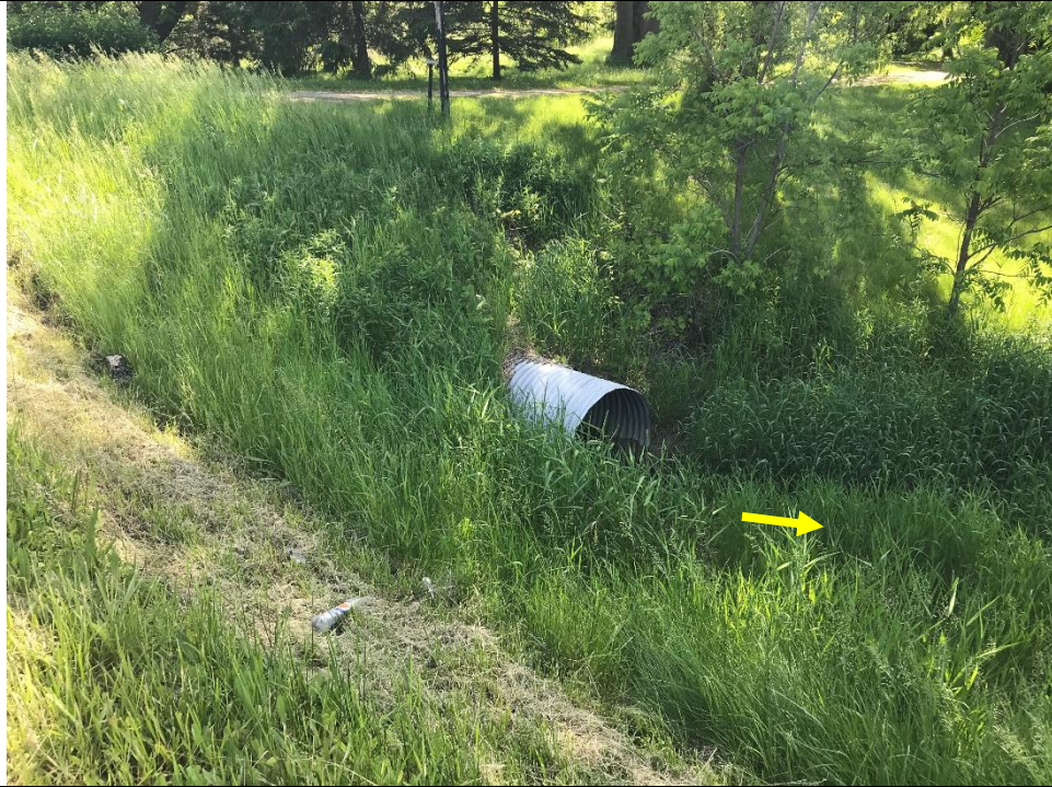
A culvert discharged flows into the feature near its downstream extent. No water was observed within the pipe during the second visit.
