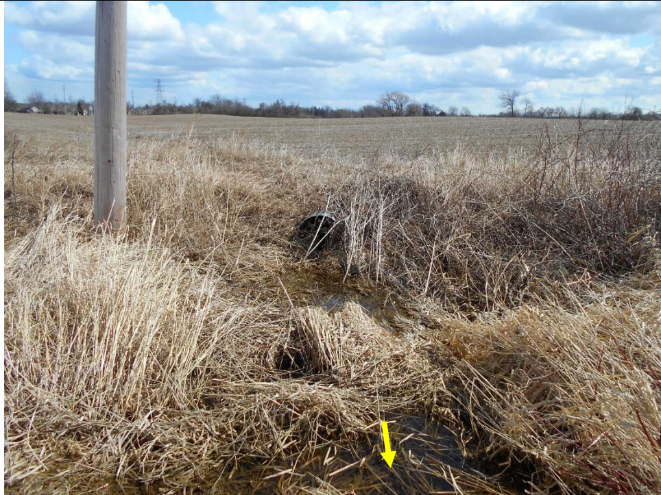
The feature had poor channel definition and originated at a culvert. The reach conveyed flows within the fallow orchard.
