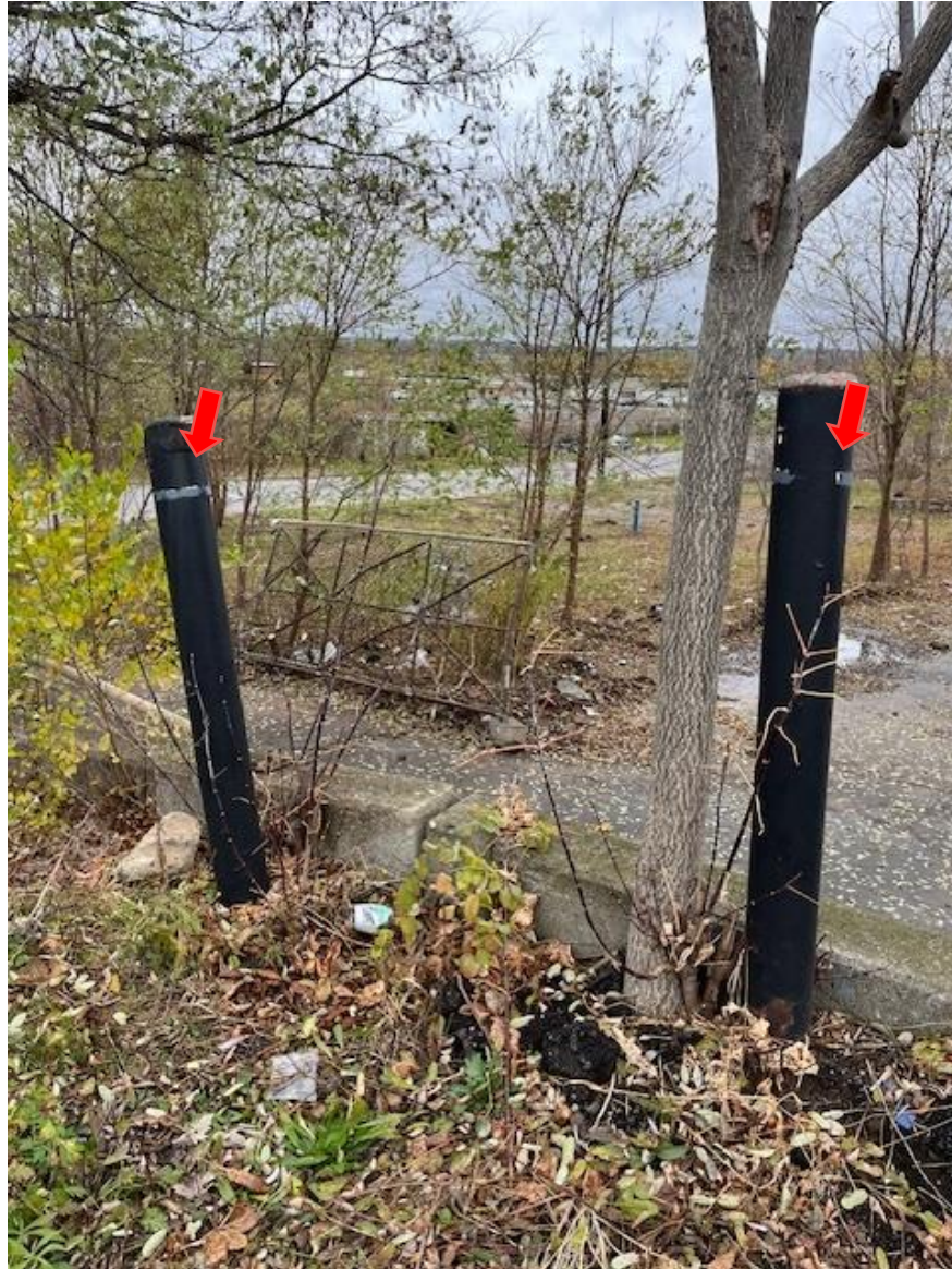
Photo 1. Representative view of lead-containing black paint applied to metal posts.
