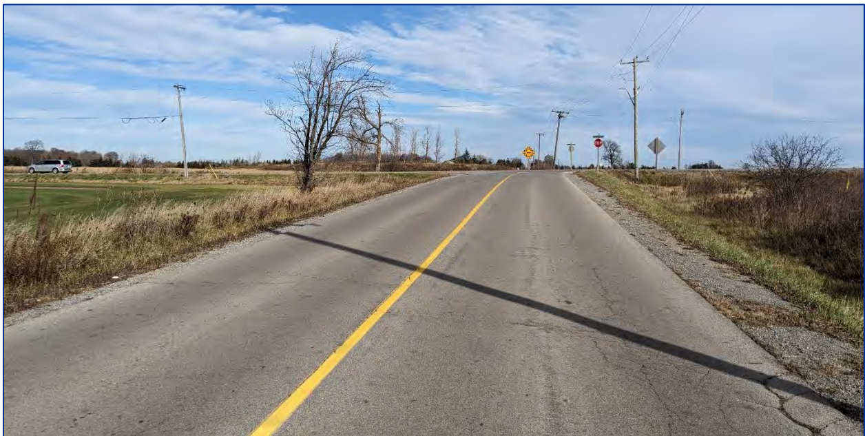
Photo 9: View looking east towards the intersection of White Church Road East and Miles Road.
