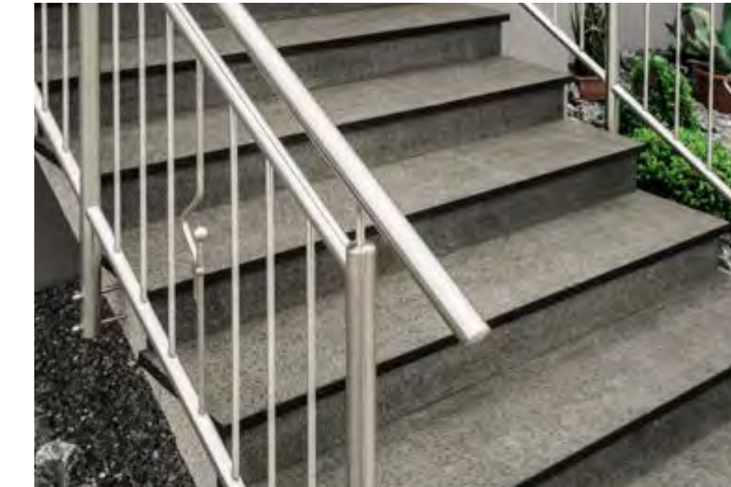
04 EXISTING STEEL STAIRCASE CLAD WITH NON-SLIP GRANITE ON BOTH TREAD AND RISER
