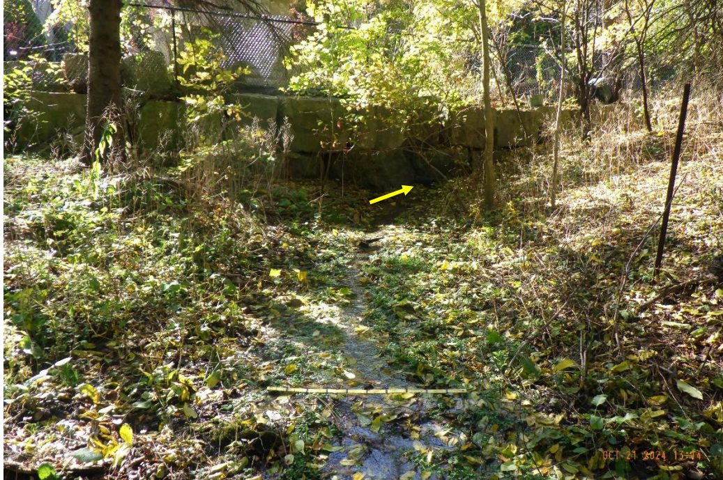
The source of the flows was observed to be from piped flows discharging from the adjacent properties.
