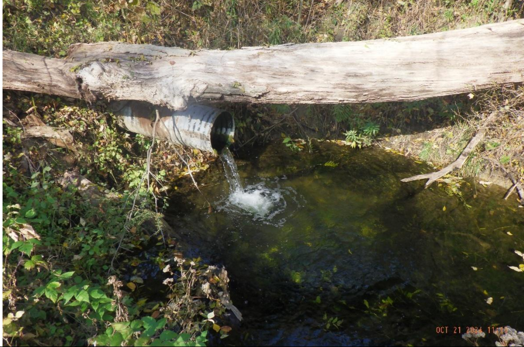
A perched outfall was present in the most upstream section of the reach with a scour pool present measuring up to 0.83 metres deep.
