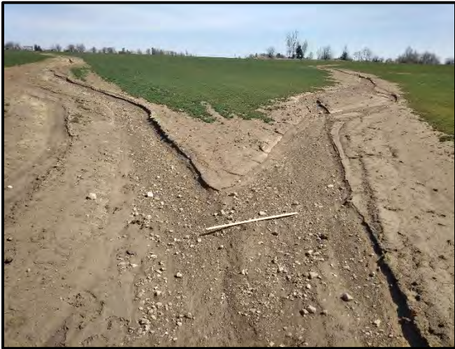
Photograph 41. Upstream View of DF15a (right) and DF15b (left) Taken at Their Confluence in Round 1. View: N Date Taken: April 16, 2024 Site: Parcel 47
